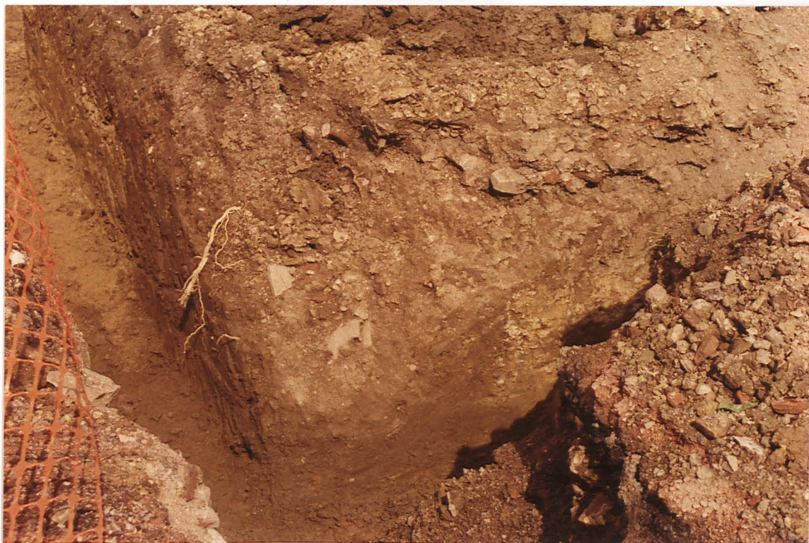
Pl. 6 Dark fill of Pit 7, visible at the corner of foundation trenches (looking NW).
