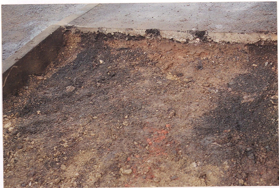
Pl. 3 The deposits exposed below the tarmac path in Market Street represented former path surfaces and back-filled service trenches.
