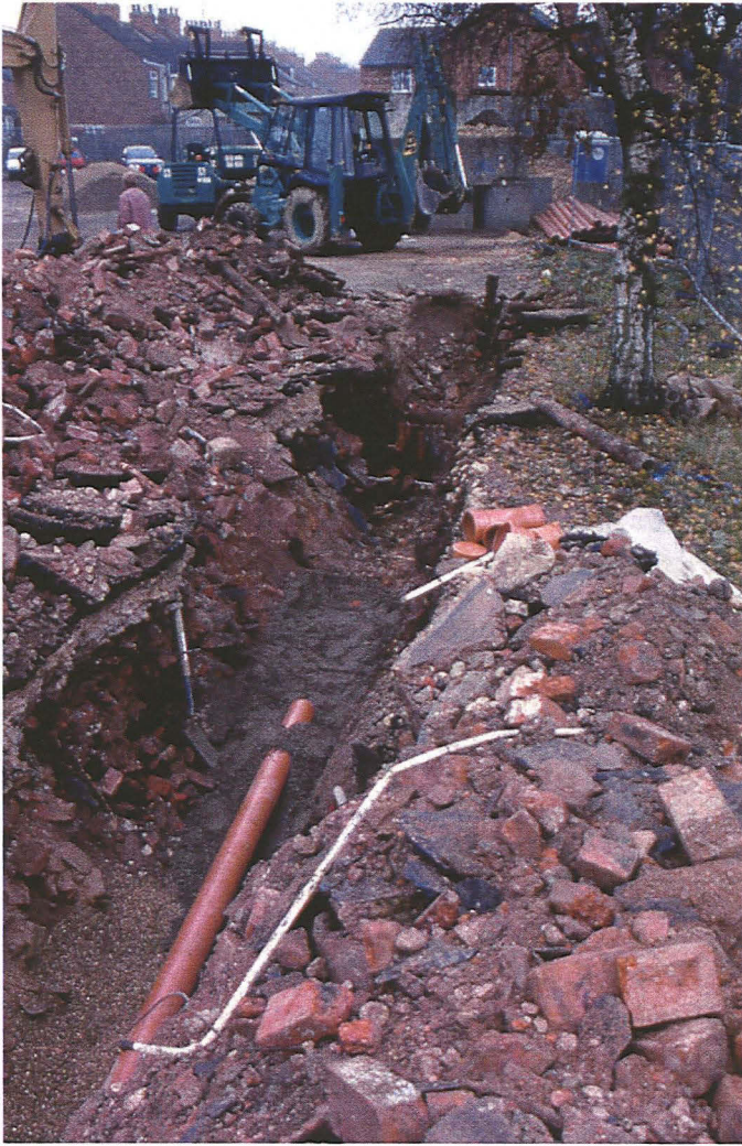
◀ Plate 1 General view the pipe trench along the South Parade site frontage looking southeast.
