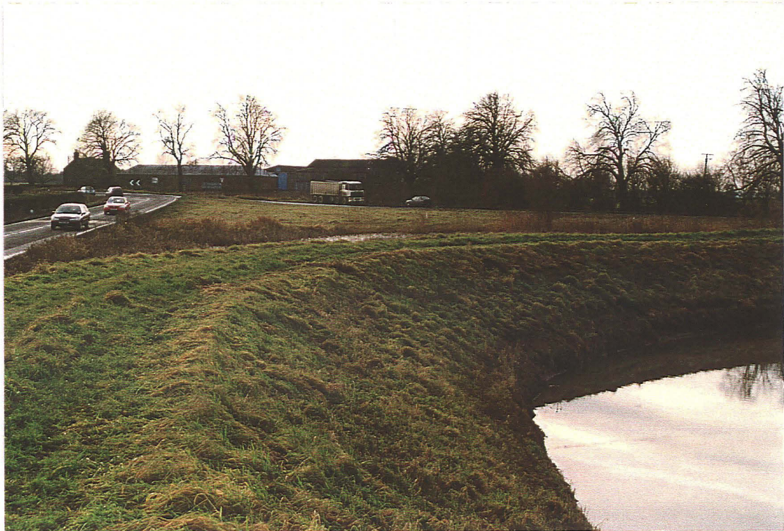
Plate 3: Section (39) - image taken from the top of the flood bank, at the pronounced bend in channel of the Billingham Skirth, looking south-west. The lorry is situated over the in-filled channel of the Car Dyke, which runs directly toward the viewer.
