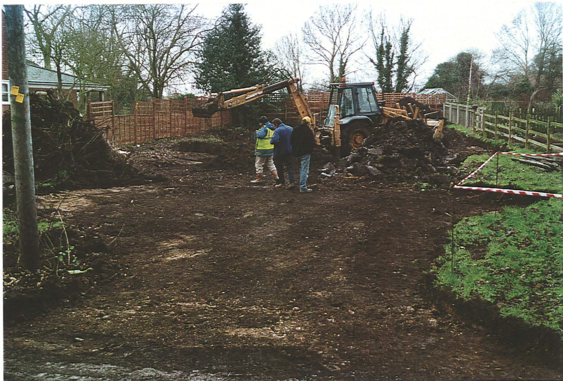
Plate 2: General view of the site during clearance works, looking NW. The JCB is parked in the area of the house footings.
