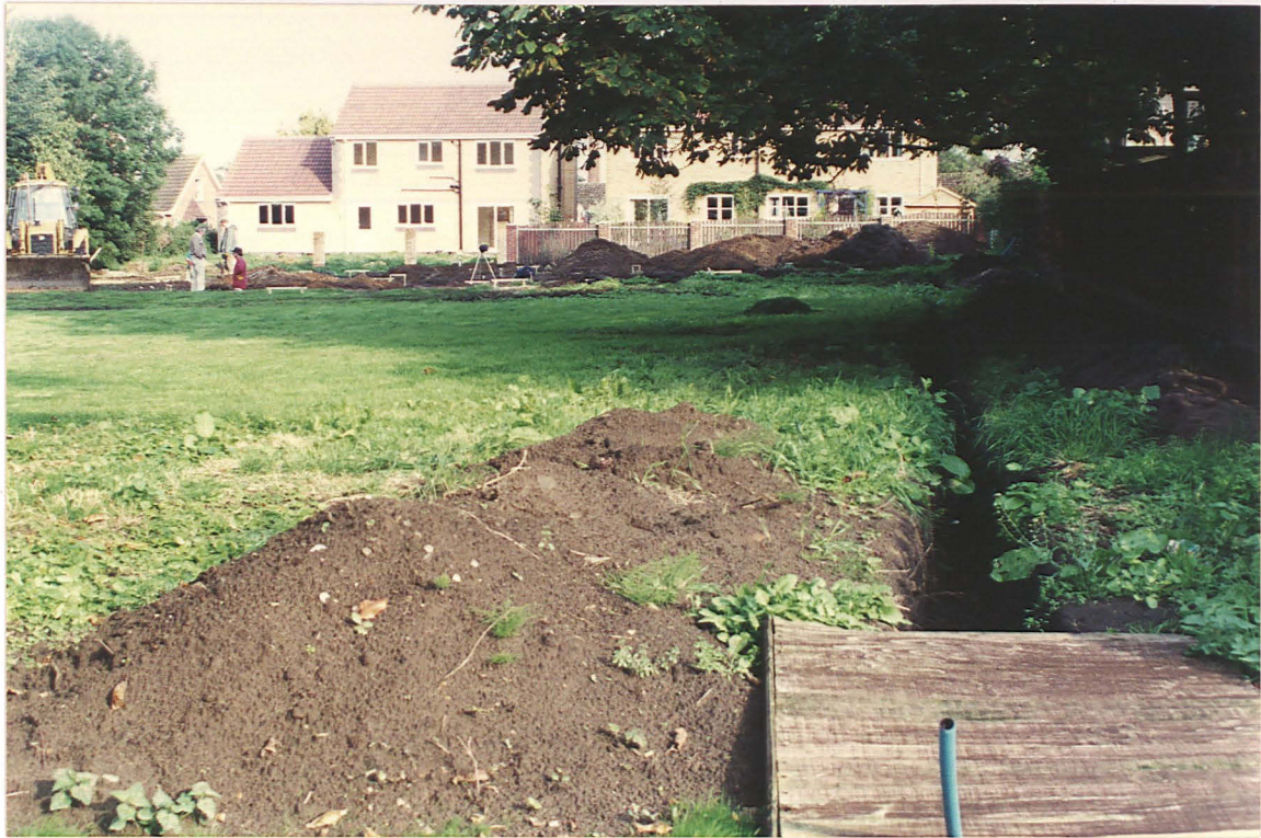
Pl. 1 General view looking east showing water pipe trench running along southern boundary of the site.
