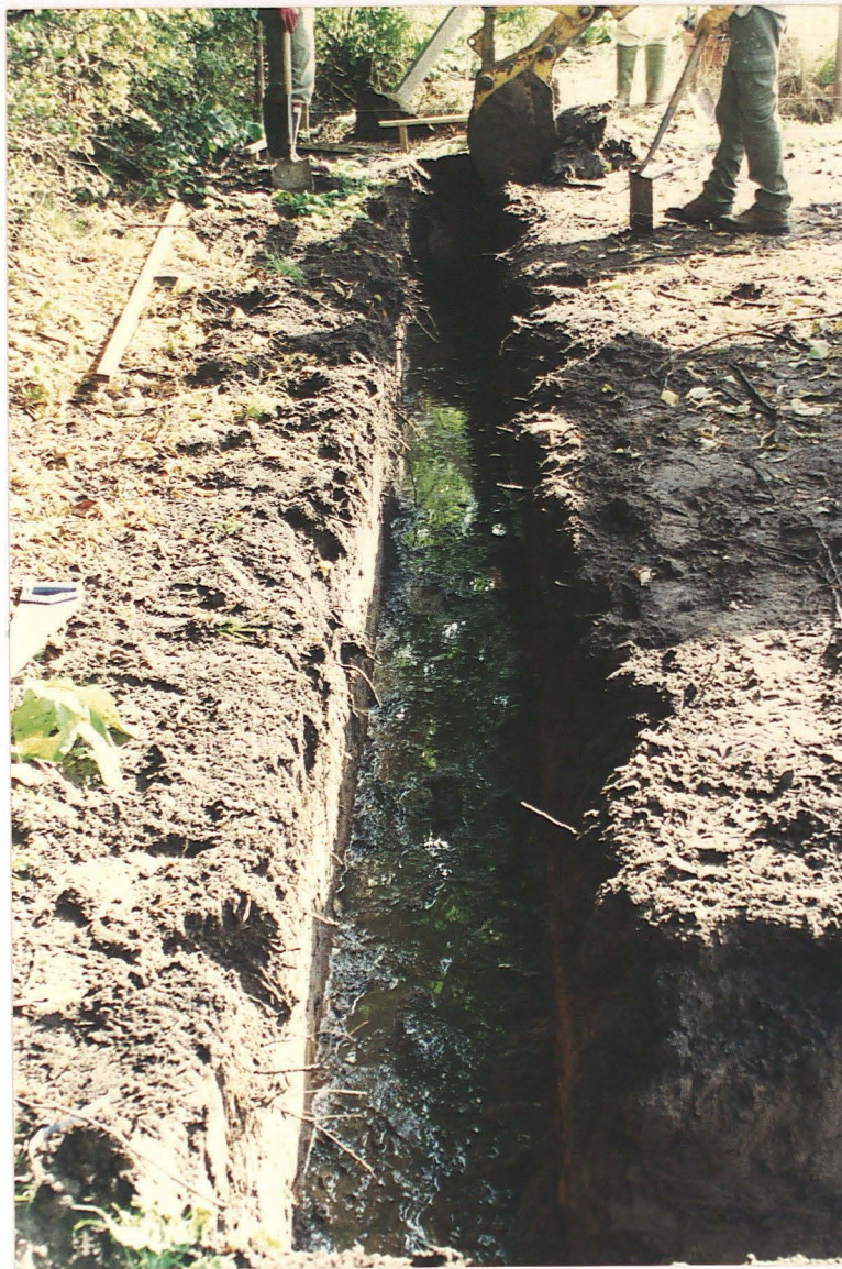
Pl. 3 North trench of the garage, looking east showing water in base of trench.
