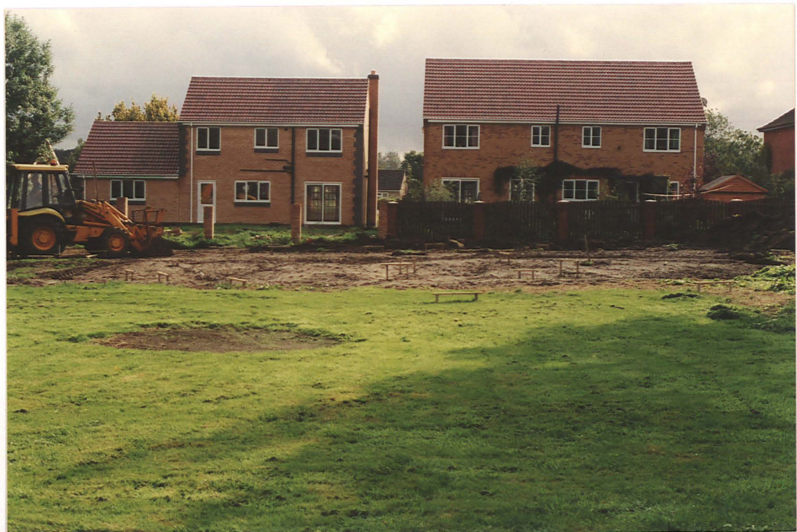
Pl. 2 General view of the house plot at the east end of the site, looking east, garage plot to left, beneath JCB.
