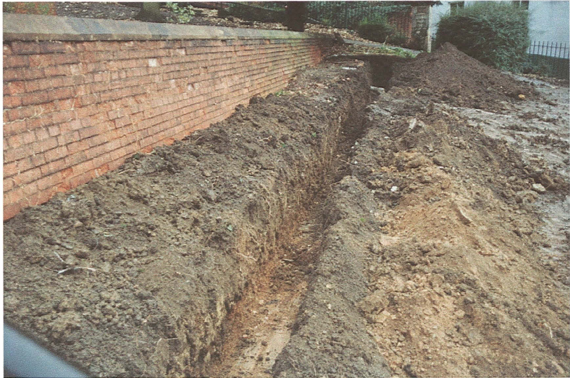
Plate 1: General view of cable trench, adjacent to terrace retaining wall - looking east
