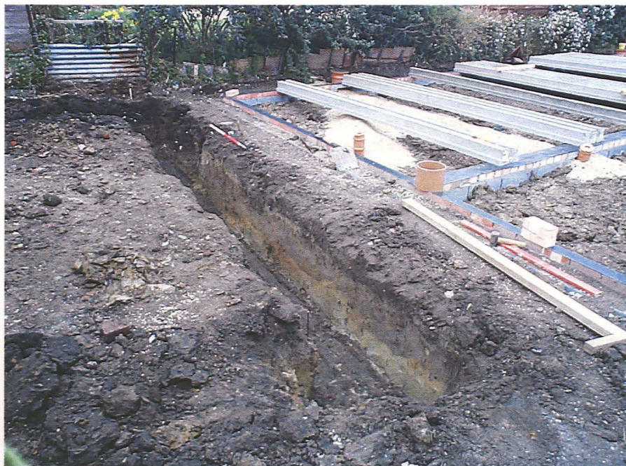
Plate 6 General view of garage footing showing oblique section through post-medieval ditch (001), looking northeast.
