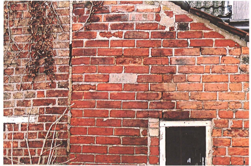
Plate 30: Detail of Phase IVB extension to No 11 showing '1957' plastic repair
