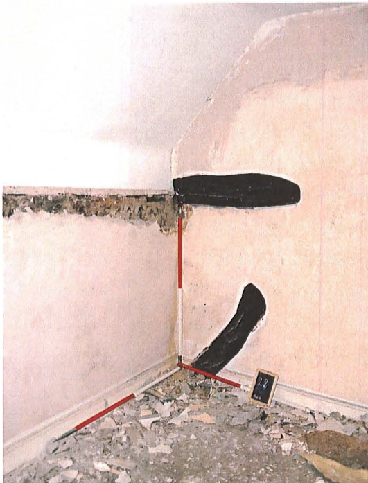
Plate 10: Blacked brace and tie-beam, Frame C, visible in east wall of Room Aii
