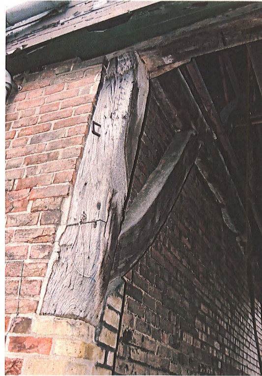
Plate 11: Frame C, principal post, brace, wall plate and tie beam showing upper-face
