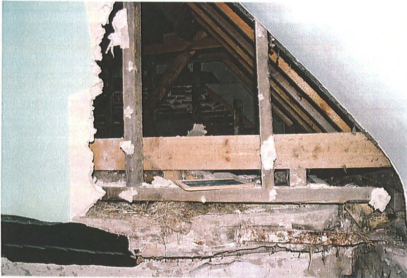
Plate 21: Rear of Phase III stud partition seen through opening-up in Room Aii
