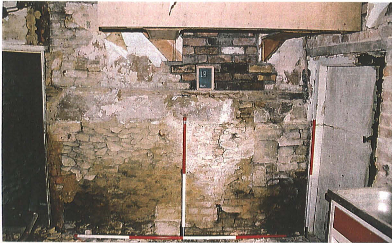
Plate 1: North elevation of Room C showing stone pinning. Stud visible above top right corner of door to Room B on the left of frame
