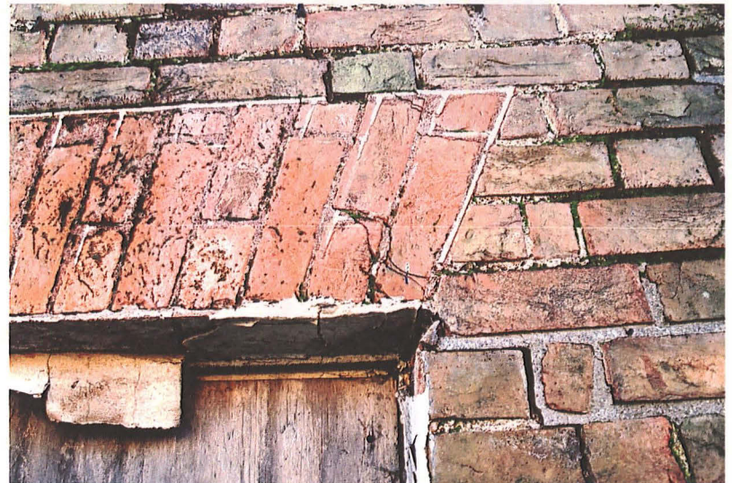
Plate 31: Detail of flat arch to window of No 9 showing tuck pointing
