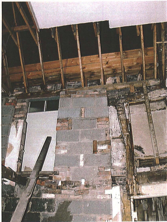
Plate 14: Room Bi, south wall, showing wall plate and stud with area of possible original infill to left of stud (partially obscured by Phase VI block work)
