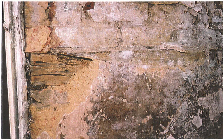
Plate 2: Detail of bridled-scarf joint to rail topping stone pinning. Doorframe of access through to Room B on the left of frame
