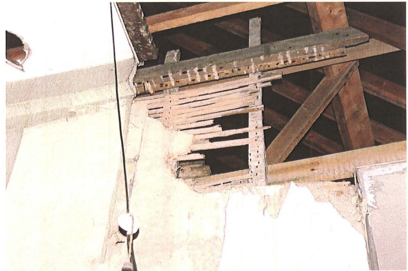
Plate 20: Room Bi; top of Phase III stud partition showing hand-split lath and plaster
