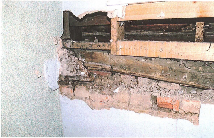
Plate 5: Wall plate and repair, southeast corner of Room Ai
