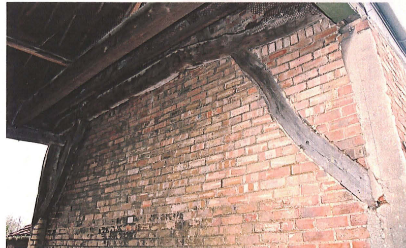
Plate 12: Frame C, frame taken from East Street showing replaced brace and tie-beam
