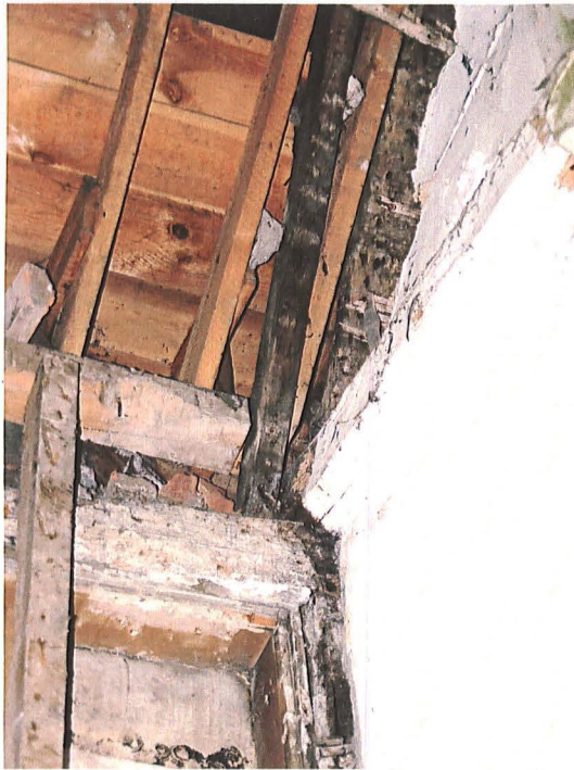
Plate 6: Room Bi, southwest corner, Frame A showing principal post, wall plate, tie-beam and probable principal rafter assembly
