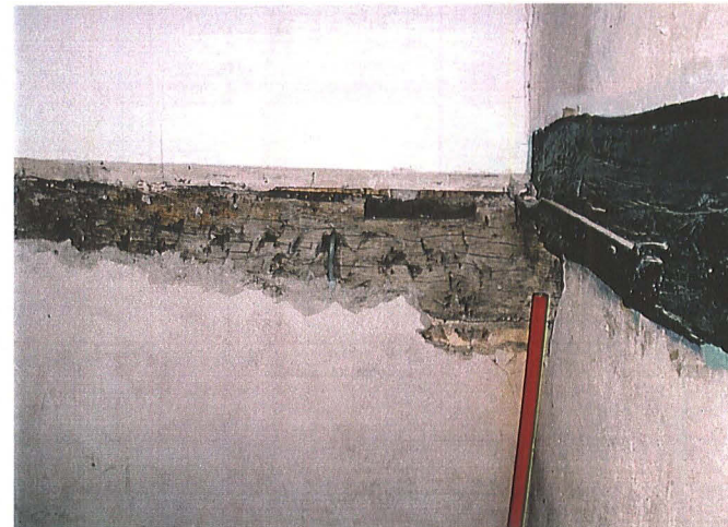
Plate 4: Frame C, internal detail of tie-beam and wall plate, northeast corner of Room Aii
