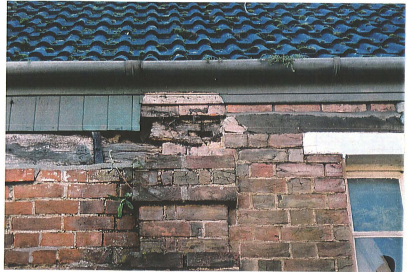
Plate 23: Detail of rusticated pier showing decayed wall plate. The timber with mortice is not in situ
