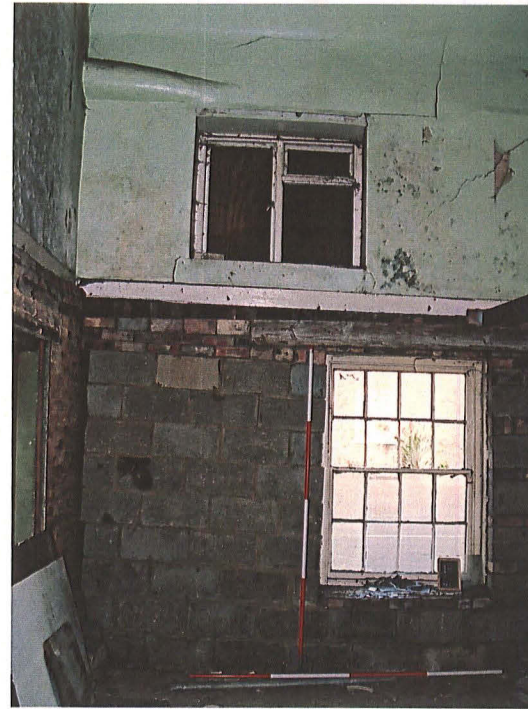
Plate 7: Frame showing bulge in the render of the northwest corner of Room Bi, indicating the possible re-use of a jowl headed post
