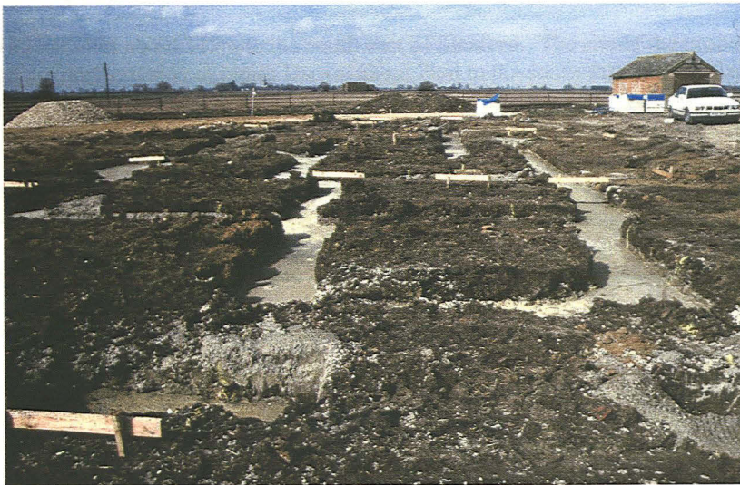
Plate 2 - View of the main development showing the infilled foundation trenches, looking west
