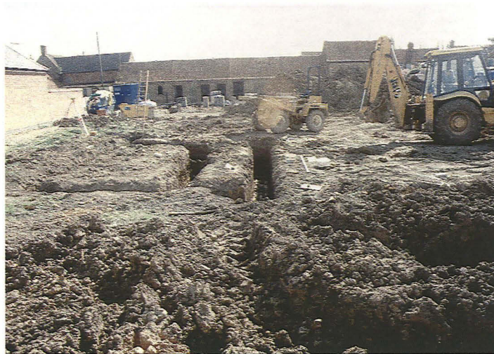
Plate 1 - General view across the development area (Plot B5 in the foreground), looking east
