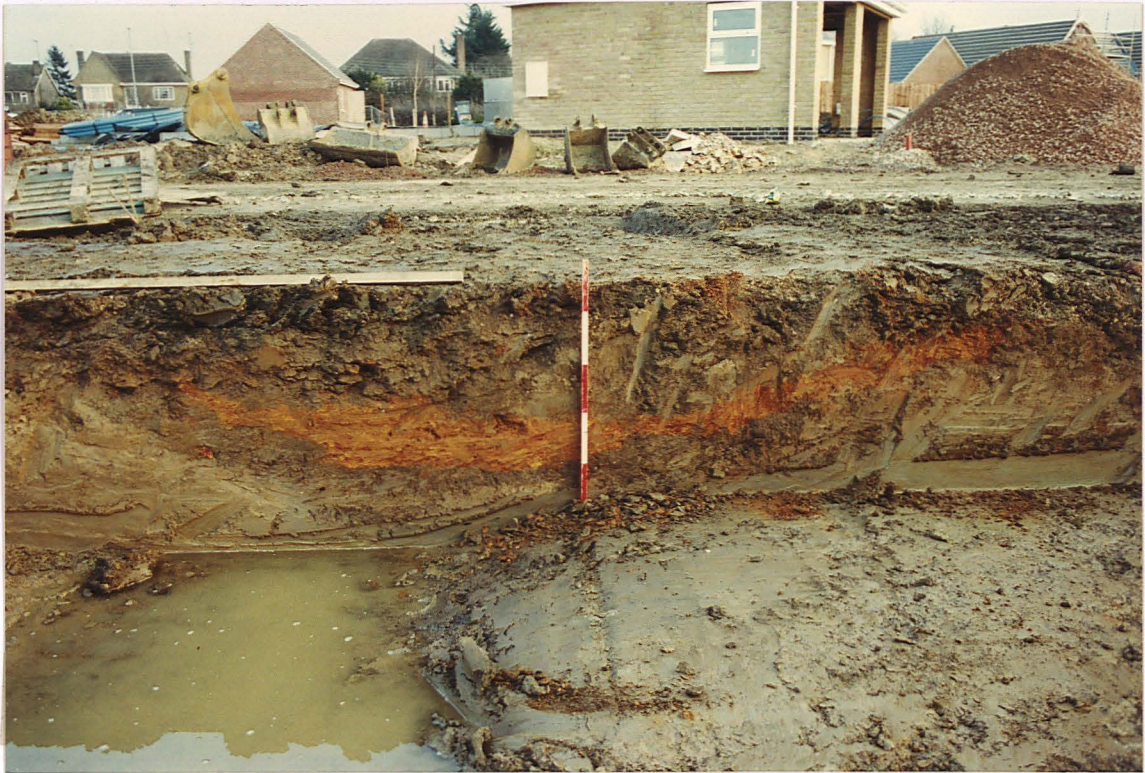
Pl. 4 House Plot 28, with red fired soil and brickdust in Ditch 172 (looking east; scale 1m).
