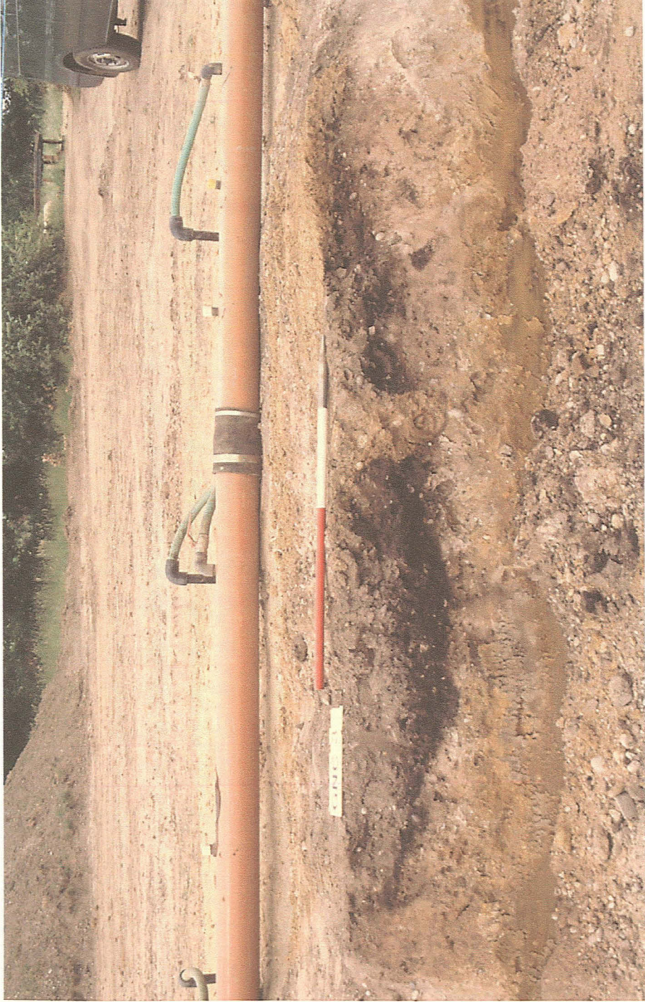
P1.3 Ditch 0200 and land drain 0204 within west section of Area 5 pipe trench. Photo by R. Holt.
