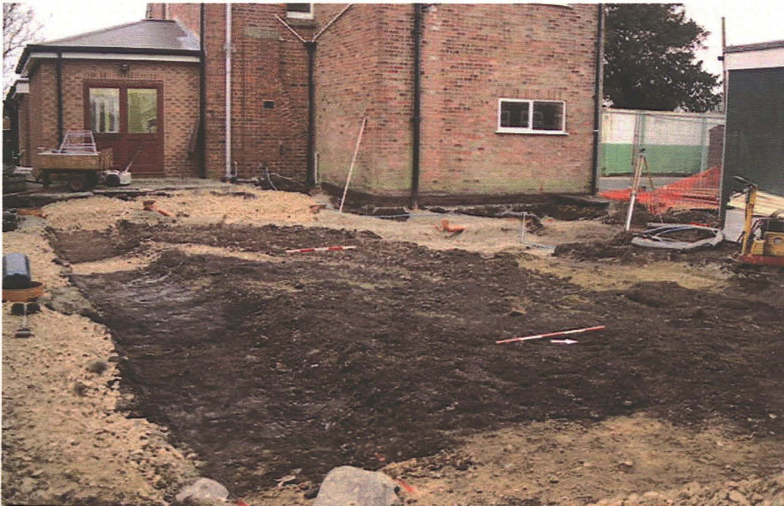
Plate 4: General view of the site after levelling and excavation of the blindings trenches, looking west.
