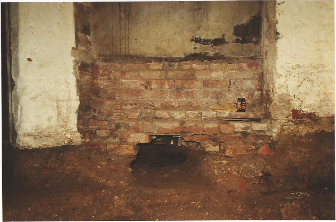
Pl. 9 Blocked tower west door, with hole for services. Base of hole is original threshold level for the door.
