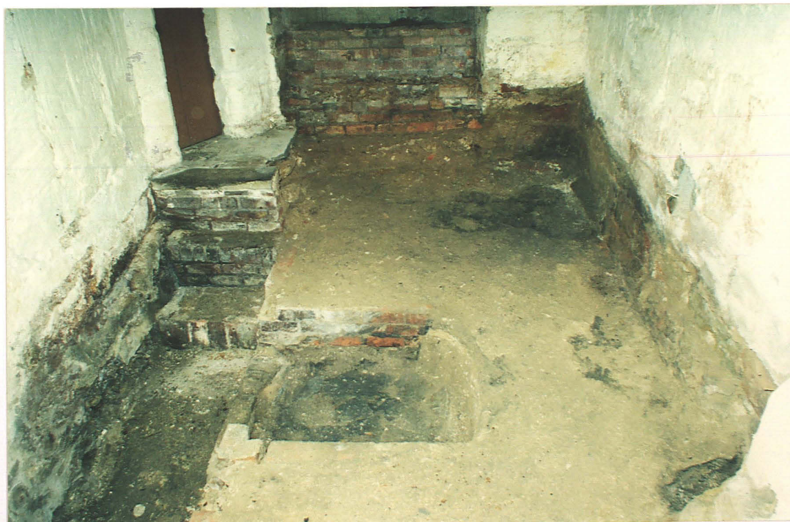
Pl. 2 Tower interior after removal of rubble beneath floorboards, looking west. Note brick steps leading to boiler, left and coal bunker in centre of floor. Area of burning in top corner may indicate position of stove.
