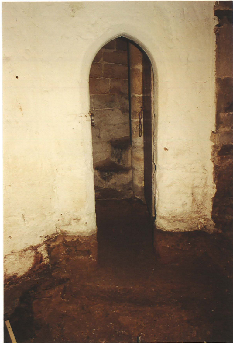
Pl. 4 Doorway and threshold to stair turret after removal of boiler house steps.
