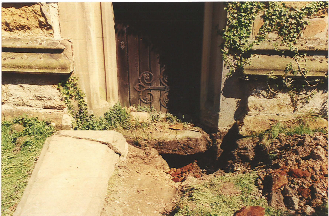
Pl. 12 Tower west door after excavation for services. Note iron hinge, copy of older hinge above.
