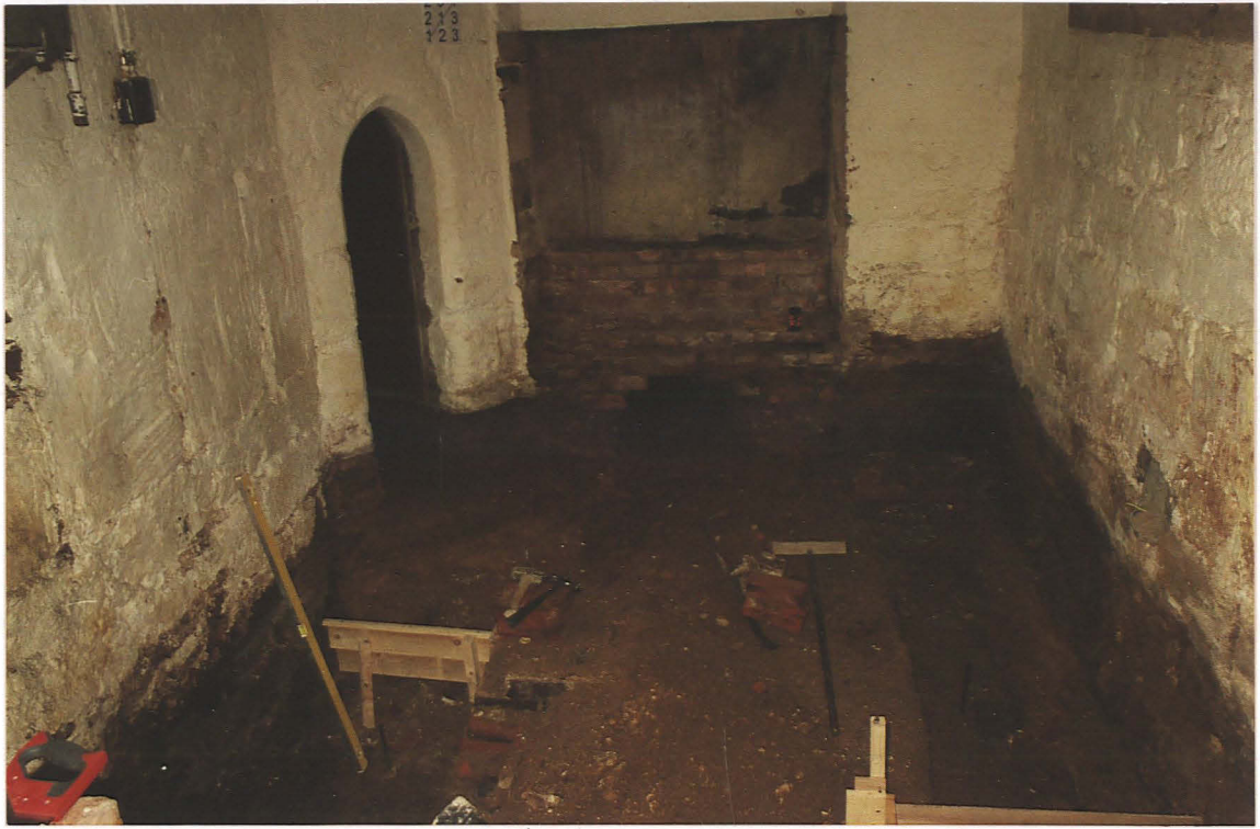
Pl. 3 Tower interior after removal of brick steps, revealing original threshold to tower stairs, looking west. Trench for services has been dug out along north wall (right).
