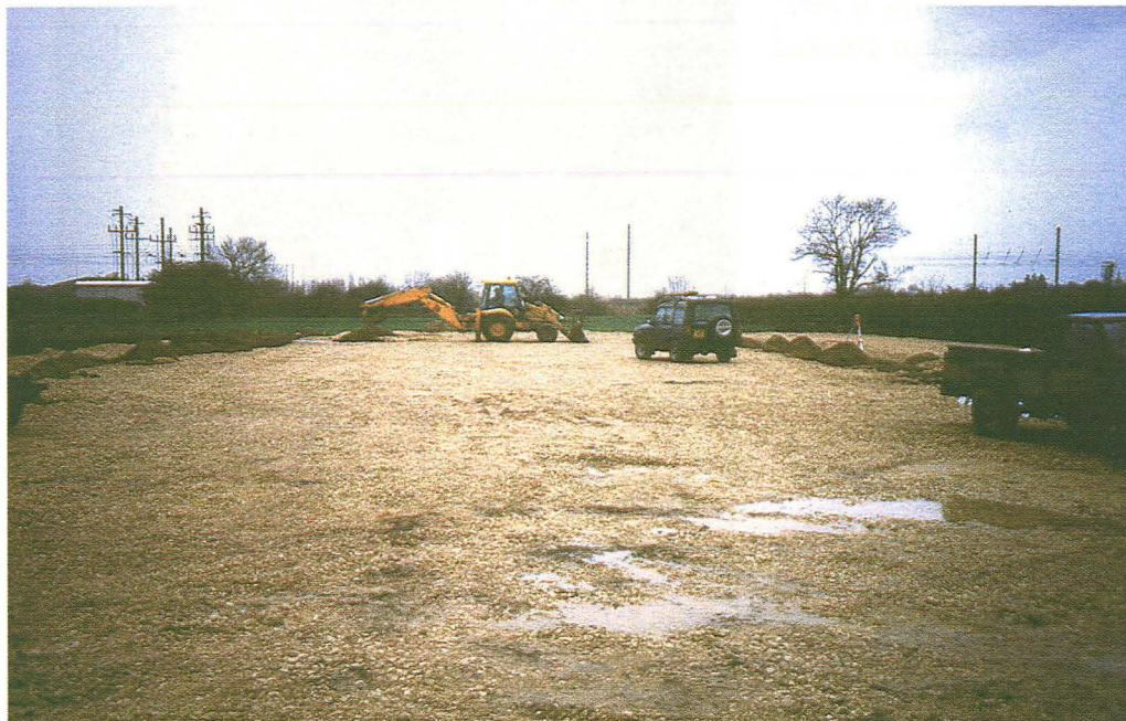
Plate 1 General view of Area A showing excavation of the stanchion pits, looking northeast.
