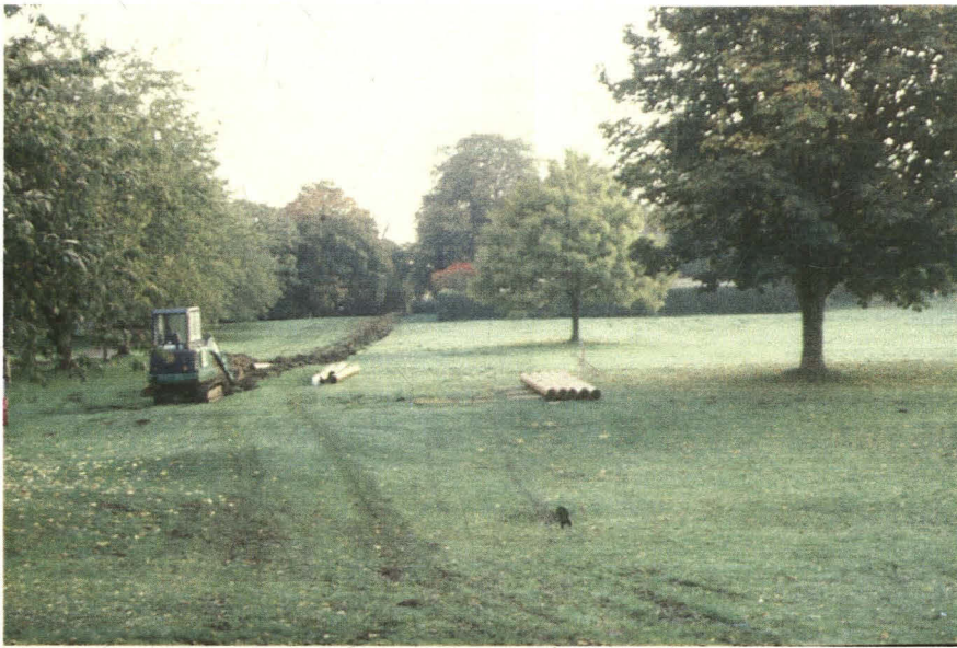
Plate 1 - General view across Bourne Castle showing the route of the pipe trench, looking north-east
