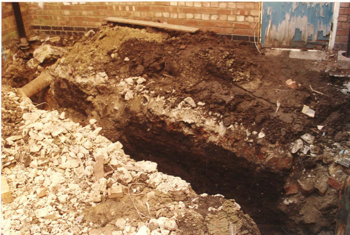
Pl. 15 Trench excavated at the western side of the Central Access Area (looking west).
