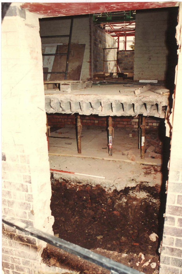
Pl. 17 Brick rubble and soil below the suspended floor in the position of the new SW Stair Access (looking west).
