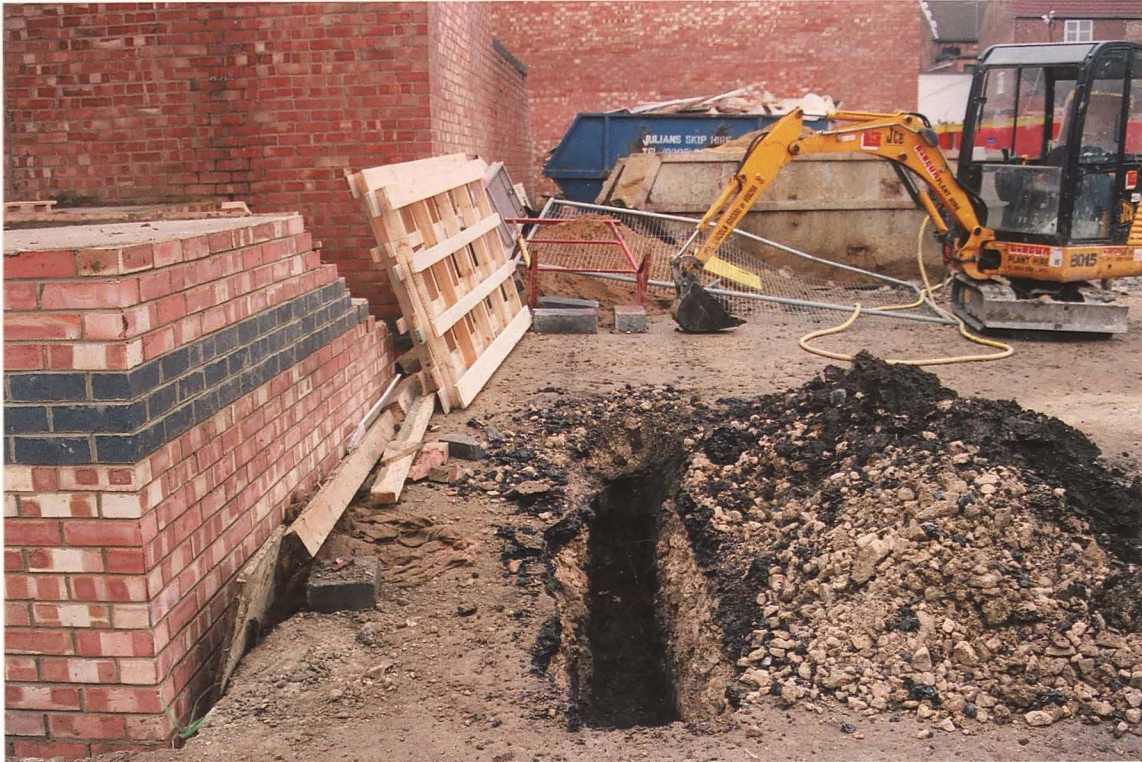
Pl. 22 Short trench excavated beside the new SE Exit (looking north towards the new extension).
