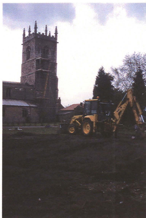
Plate 3: General view of the site during excavation of the foundation trenches, looking SW. The proximity of the church to the site is clear from this shot.
