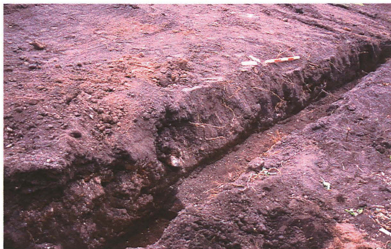
Plate 4: Brick wall foundation [012], seen in the foundation trench for the north wall of the house, looking SW
