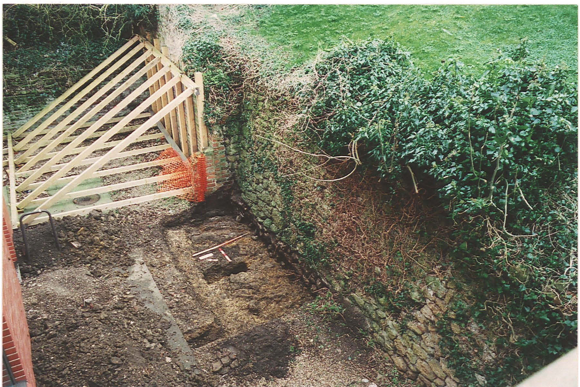
Pl. 6 Retaining wall 111 with all courses of stonework exposed. Looking east. Scales 0.50m and 1m.
