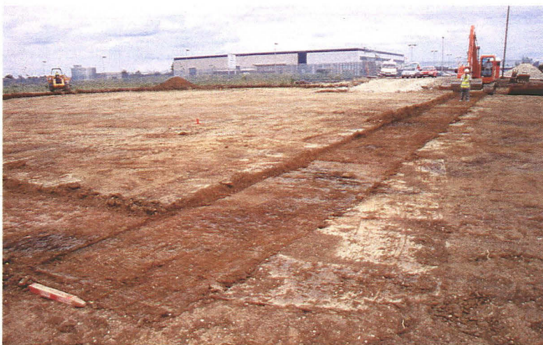
Plate 3 - View showing the removal of the subsoil (002) within the footings of the new building, looking southeast
