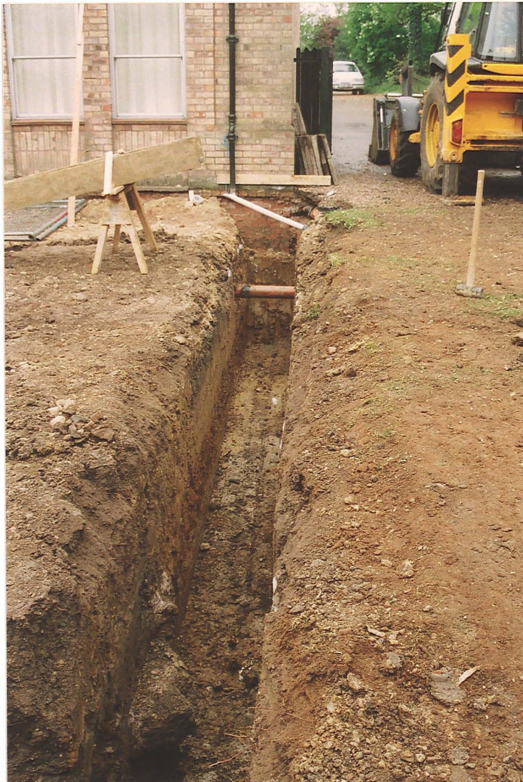
Pl. 3 Western foundation trench, with the modern concrete backfill 22 in the NW corner (left foreground). Looking south.
