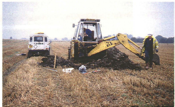
Plate 2: Excavation of Test Pit 68 in progress. Note mound of Goll Grange on left of picture.
