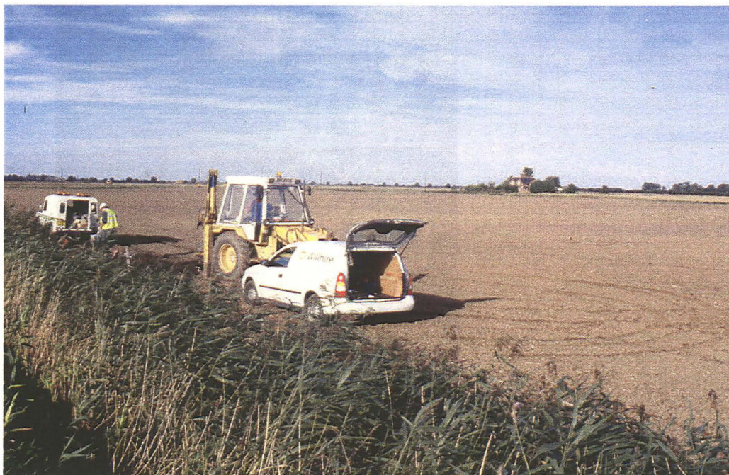
Plate 3: Excavation of Test Pit 67 within 'clay with roddons' zone in progress. Note band of lighter silts defining roddon in background.
