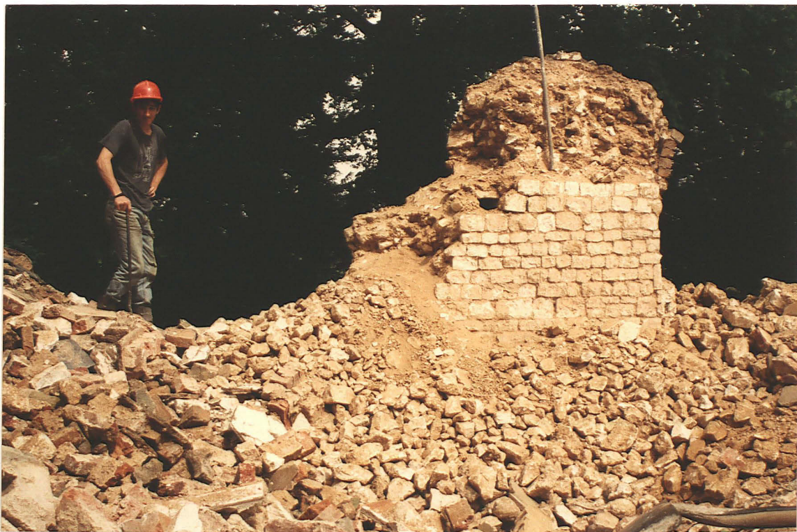
Pl.17. Nave north wall (interior), showing chalk coursing, putlog hole and rubble core.
