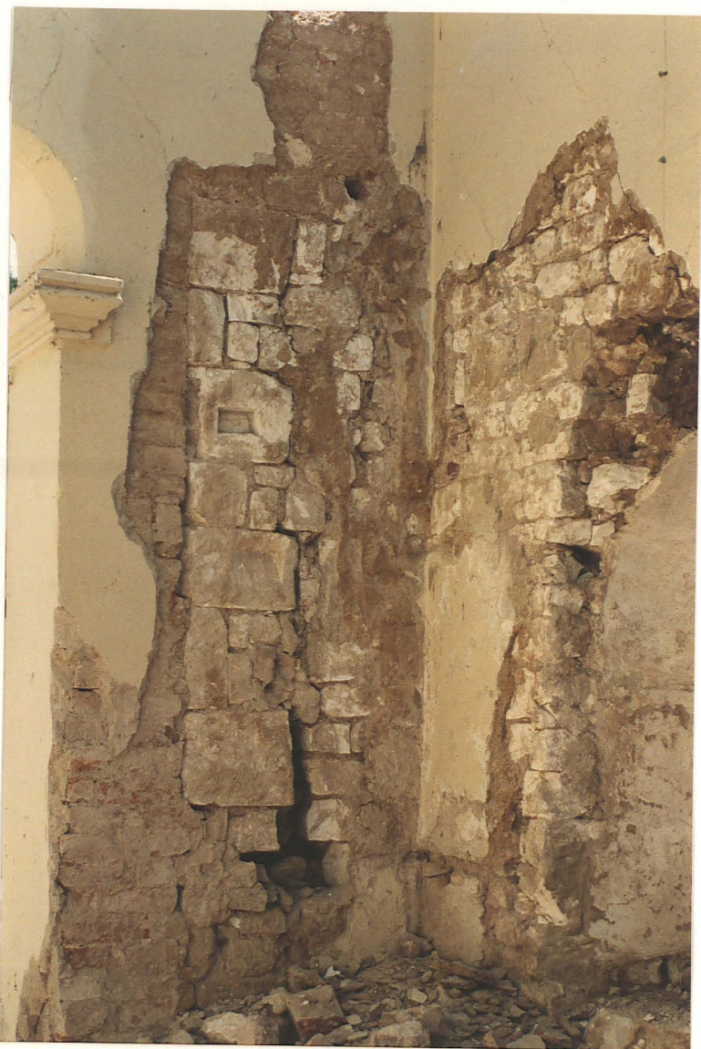
Pl. 27. South side of chancel arch showing brick facing of new arch. Note brickwork above the chalk and re-used chalk block.
