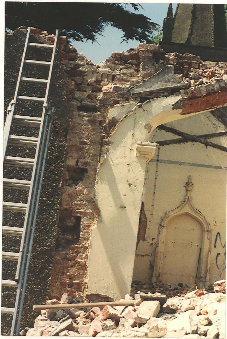
Pl. 30. Chancel arch. Detail of south side showing bonding with the chancel wall (demolished).
