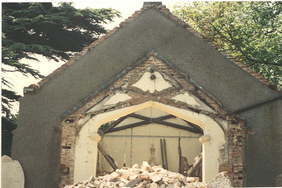
Pl. 29. Chancel arch looking towards nave after demolition of chancel. Note complete absence of any chalk and bonding for the chancel walls.
