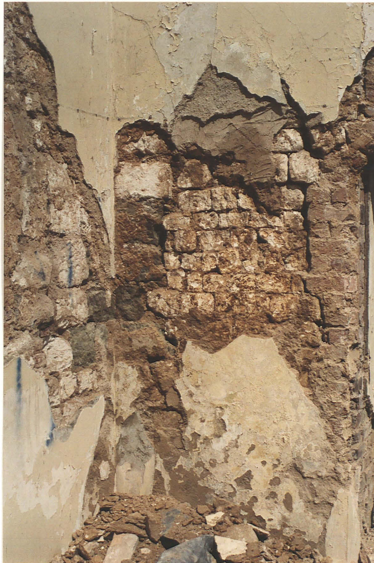
Pl.19. North west angle of nave showing later sandstone and chalk repair, original chalk wall and inserted brickwork of vestry door (right).
