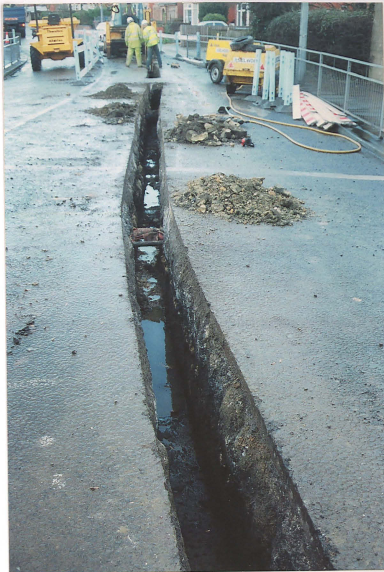
Pl. 13 Open-cut trenching in Rookery Lane (looking north). Deposits close to the junction with Newark Road (21) were dark silts, with overlying brown loam.
