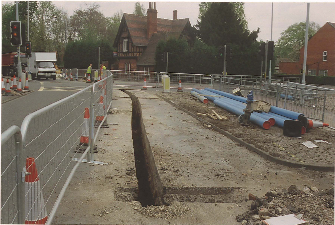
Pl. 2 At the approach to the eastern side of the river bridge (3), the foundation bedding for the modern road was thicker, with limestone rubble over clinker, ash and brick rubble (looking east).
