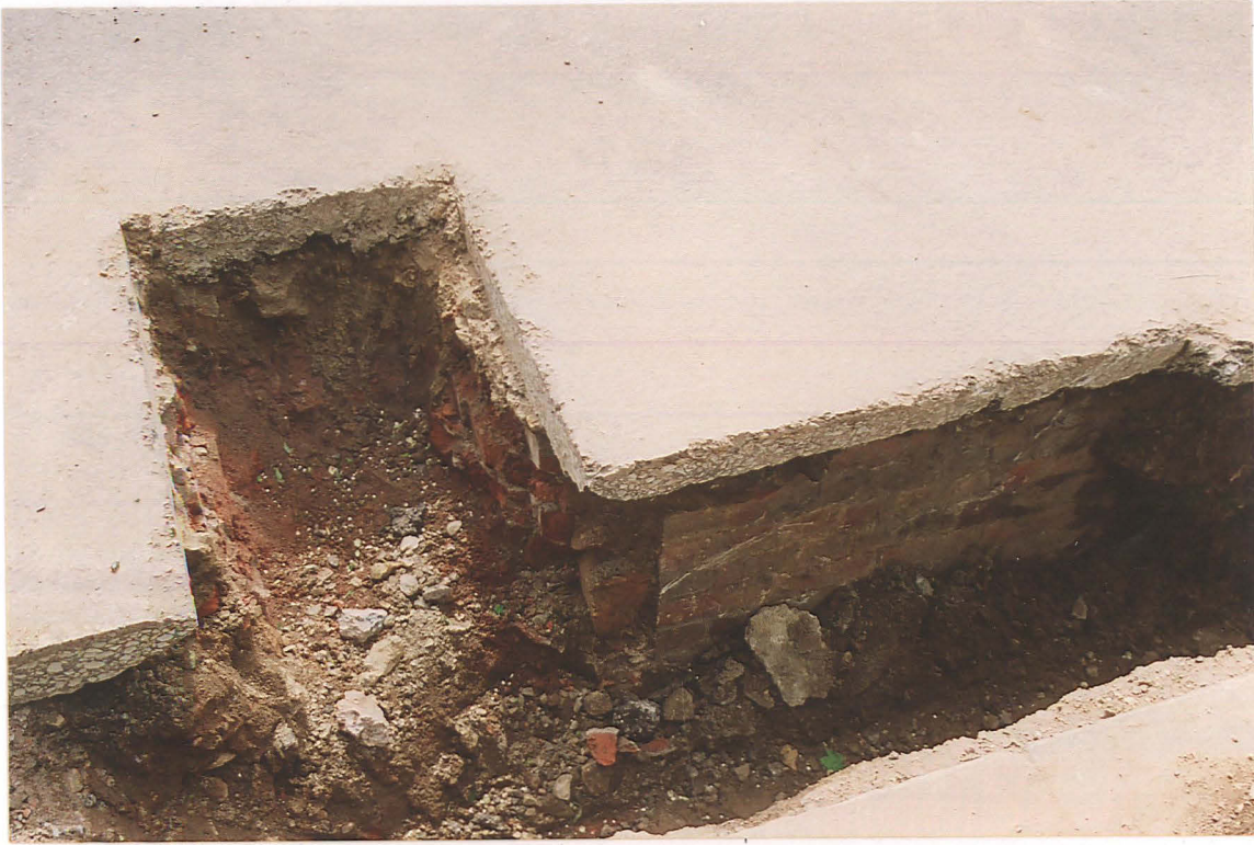
Pl. 11 Close to the junction of Doddington Road with Newark Road (15), a brick structure was seen. This is probably a bridge across the Pike Drain.
