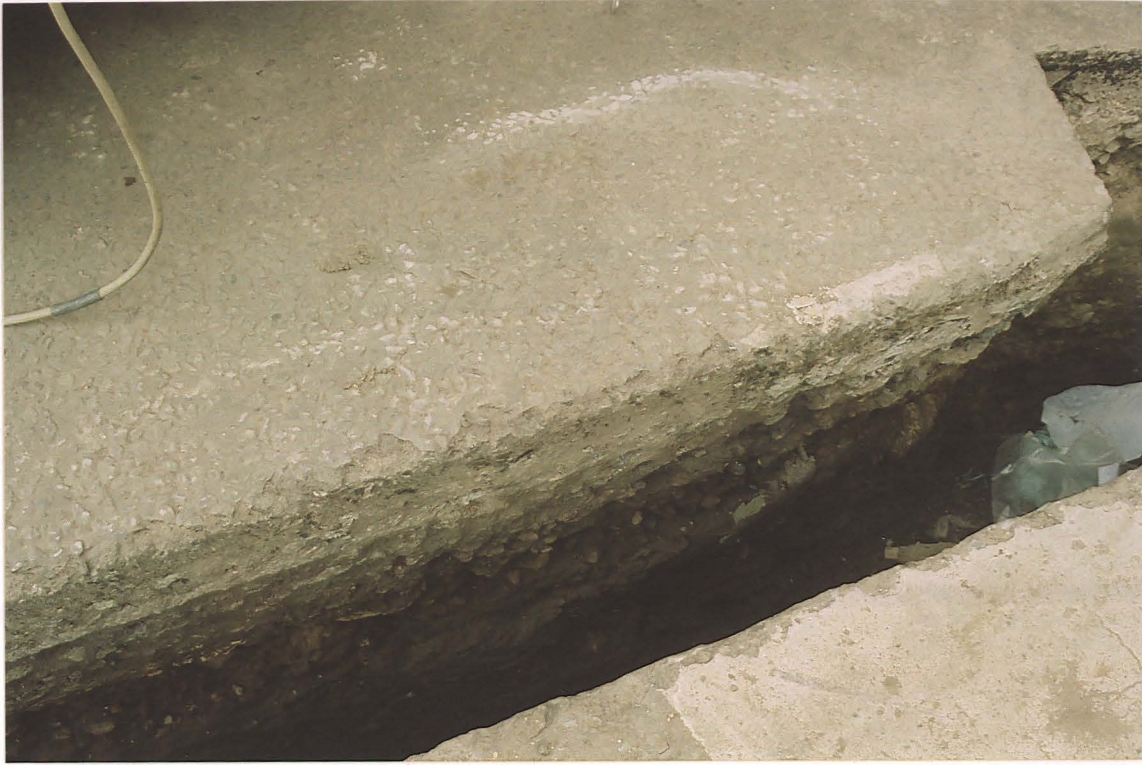
Pl. 1 The tarmac road surface overlies a gravel band near 210 Newark Road (2), probably a post-medieval road surface.
