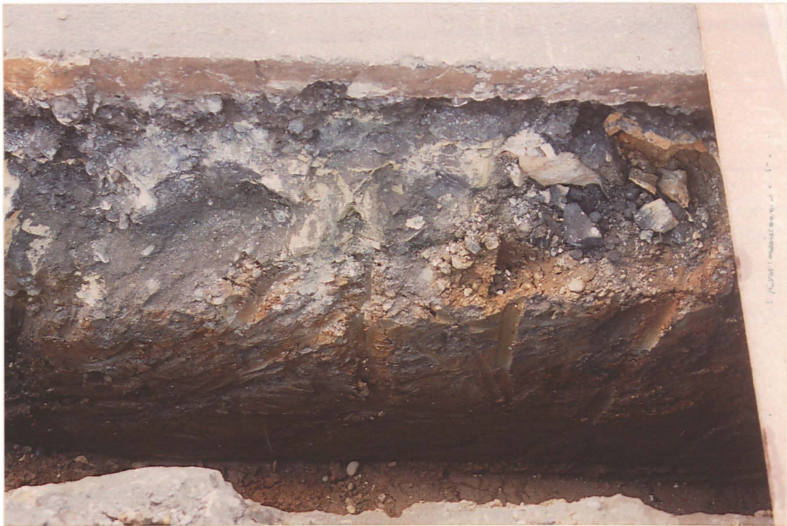
Pl. 16 The thin gravel band was traced northwards to 16 Rookery Lane (26), where it overlay clay. This suggests that the uppermost gravel may have been a post-medieval road surface.
