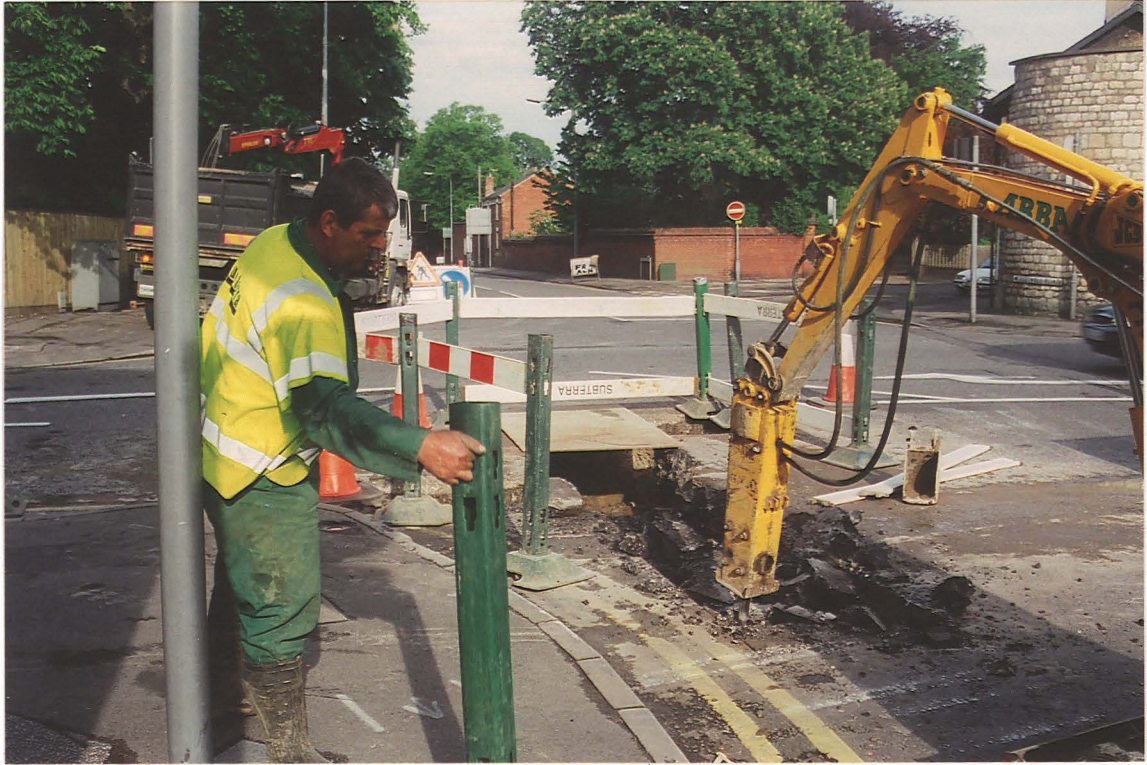
Pl. 3 Location of the Anglian Water trench (2) at the junction of Greetwellgate and Wragby Road (looking east).
