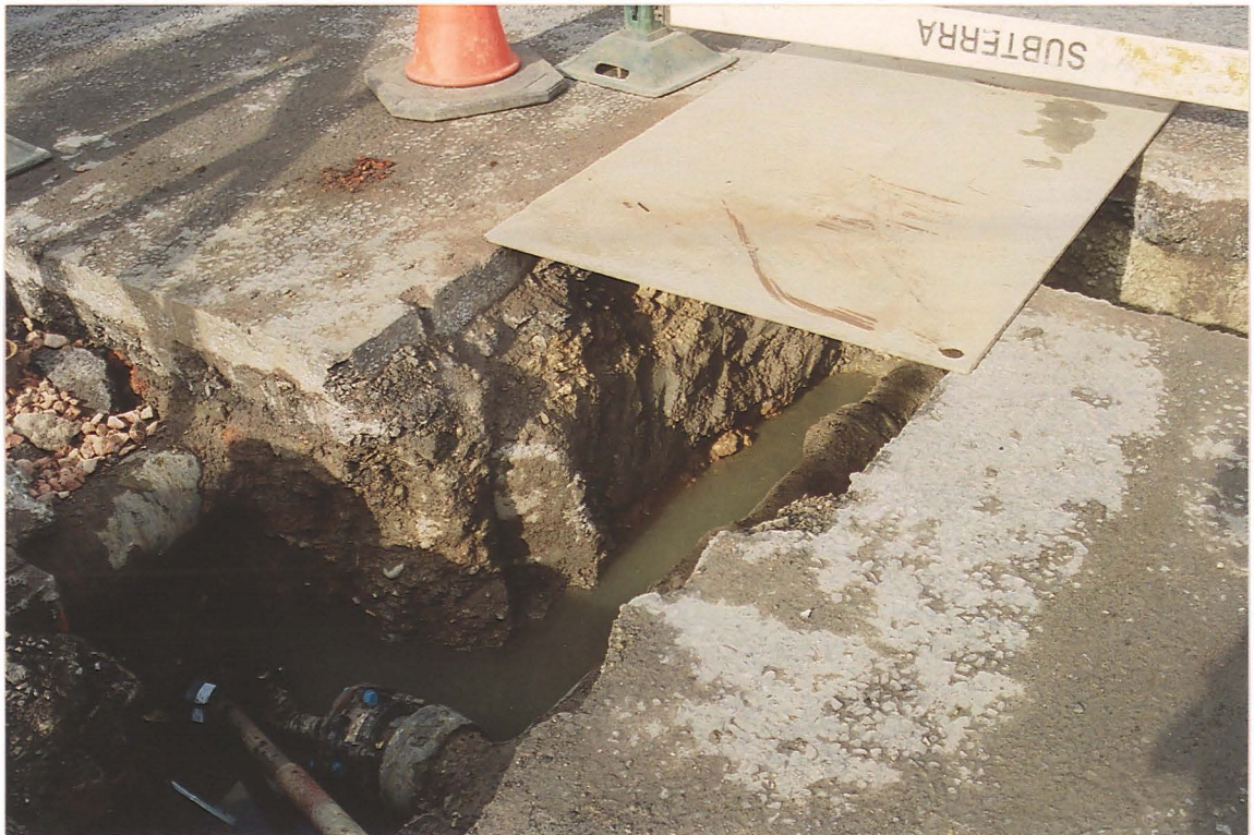
Pl. 4 Compacted gravel deposits cut by later service pipe trenches at the junction of Greetwellgate and Wragby Road (2), looking NE.
