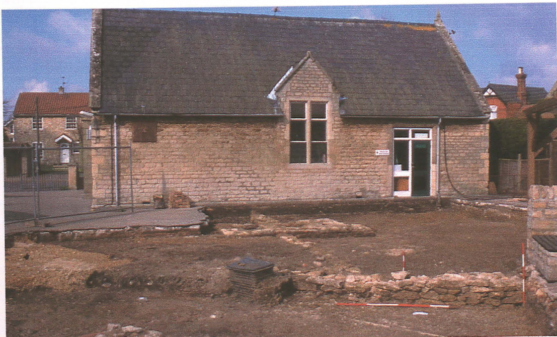
Plate 4: Area 1, showing the relationship between the toilet block, (1000), and the original school building, which only extended up to the fire door at the northern end of the wall, looking west. Wall (1008) is visible bottom right.
