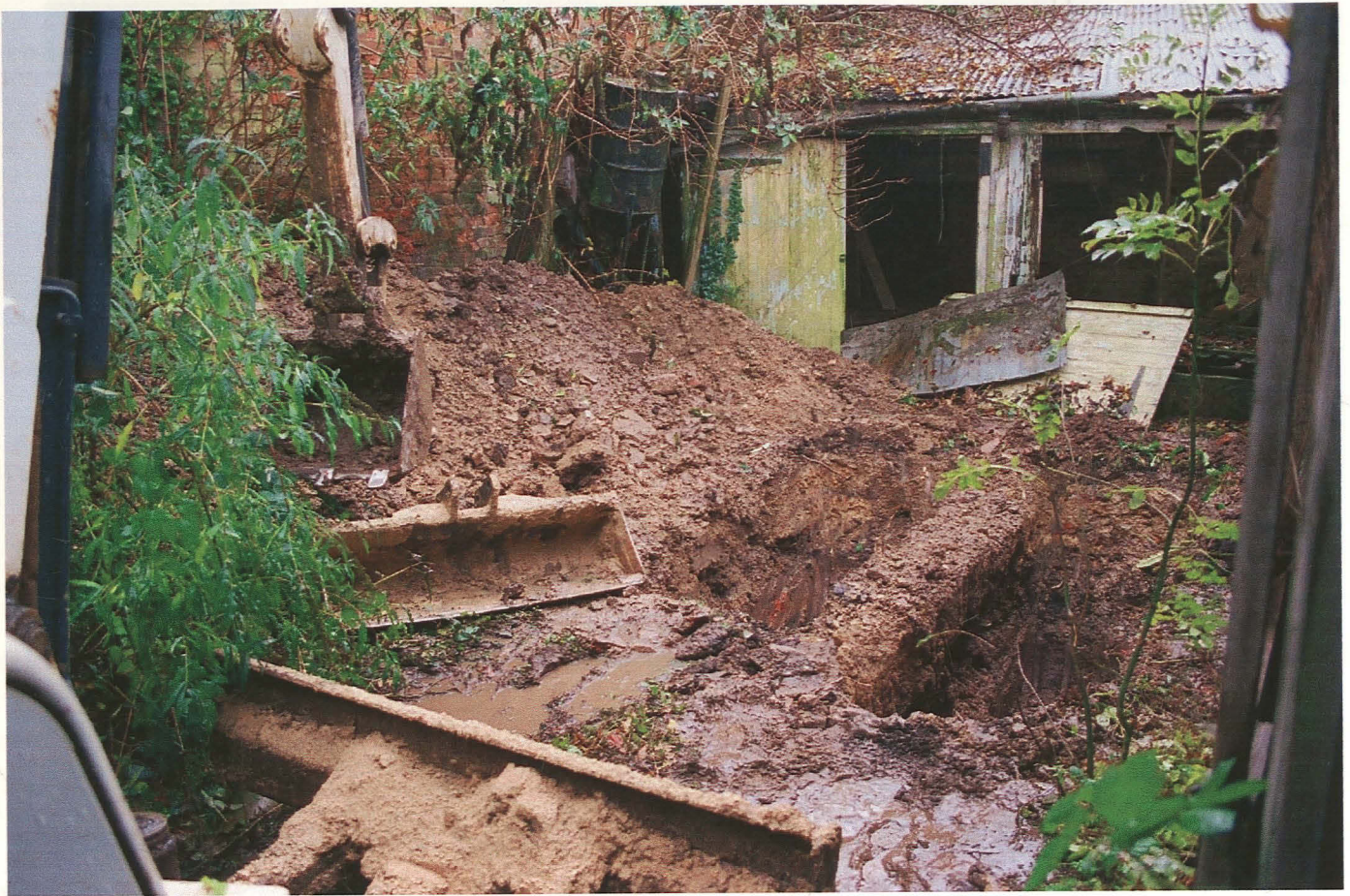
Pl. 4 General view of trench with sewer pipe running through centre, looking southeast.
