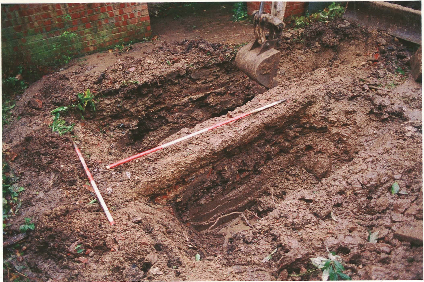
Pl. 6 General view of trench with sewer pipe running through centre, looking southeast.
