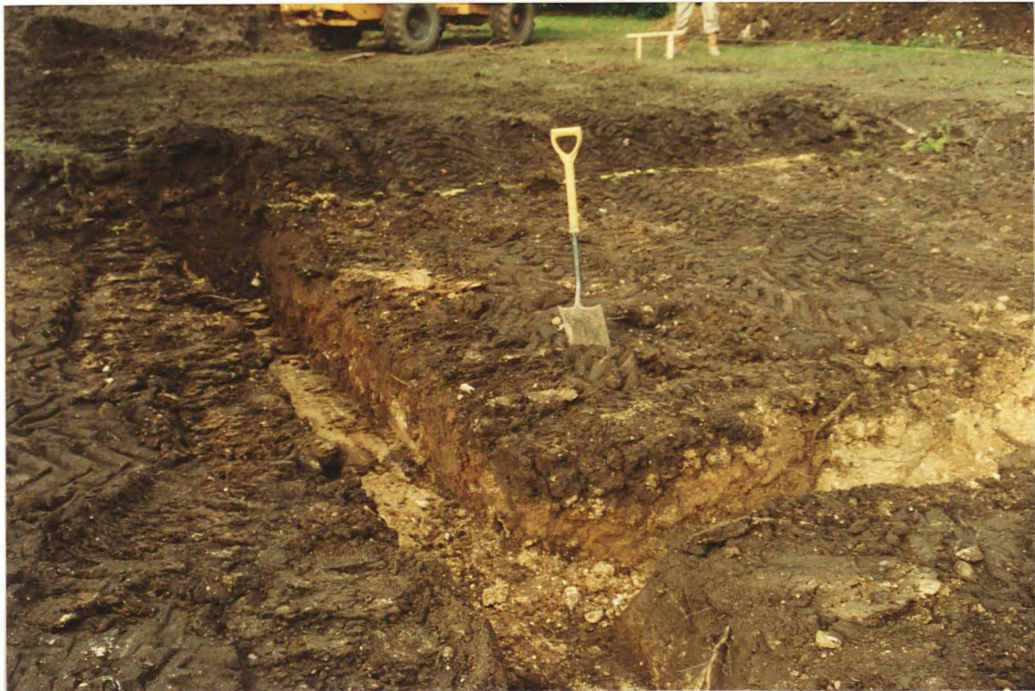
Pl. 7 Foundations for the bedroom, showing the orange clay fill of pit or ditch 29 (looking NE, with well 30 in the top left corner).
