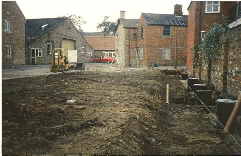
Plate 1 - General view of the development area and service trench, looking west towards Navigation House
