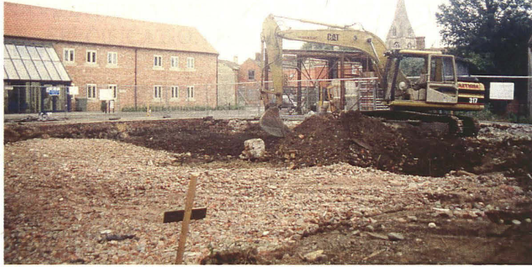
Plate 1 - General view across the development area, looking northwest towards St. Denys' church
