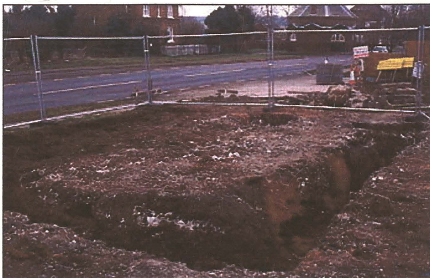
Plate 3 (left): General view of the garage plot, looking SE, with the Buttercross in the background. Two slurry-filled inspection pits for fuel tanks can be seen in the foreground.
