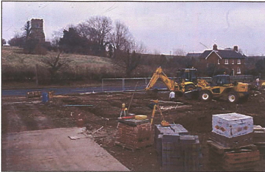
Plate 1 (left): General view of the development site, looking ESE, with St. Michael's church in the background.
