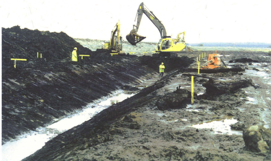
Plate 2: The new soke dyke under construction, showing the depth of the peat deposits at the north-east corner of the island, looking east.
