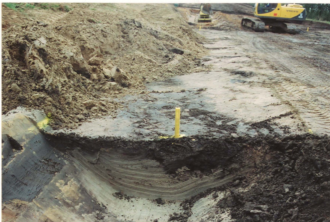
PI. 4 Dark fill at the broad, rounded base of ditch 800 showing in the deeper trench (below the peg), with the pointed base of 840 in the trench side (left). Looking south.
