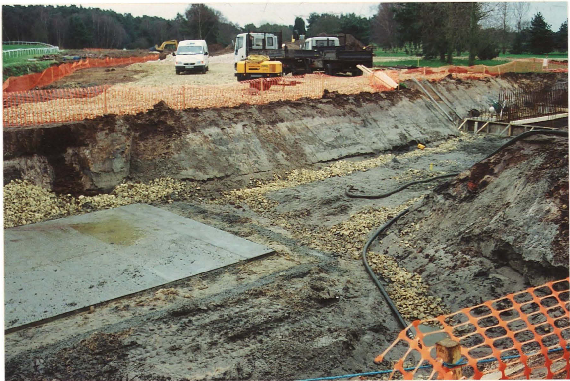
Pl. 11 Soil profile at the northern side of a trench excavated for new flood defence structures, north of the monitored area (looking NE).
