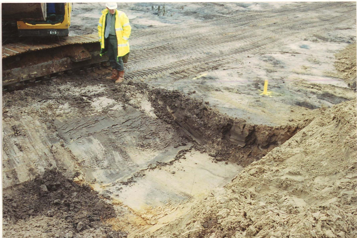
PI. 2 A deeper trench was excavated along the eastern edge of the stripped area (looking NW, with the grey fill of 836 visible in the trench sides).
