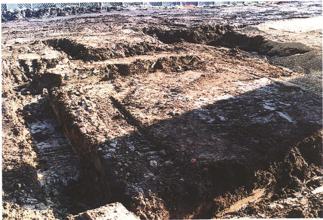
Plate 2: North-west corner of the site, after the removal of the former school foundation trenches, looking south-east
