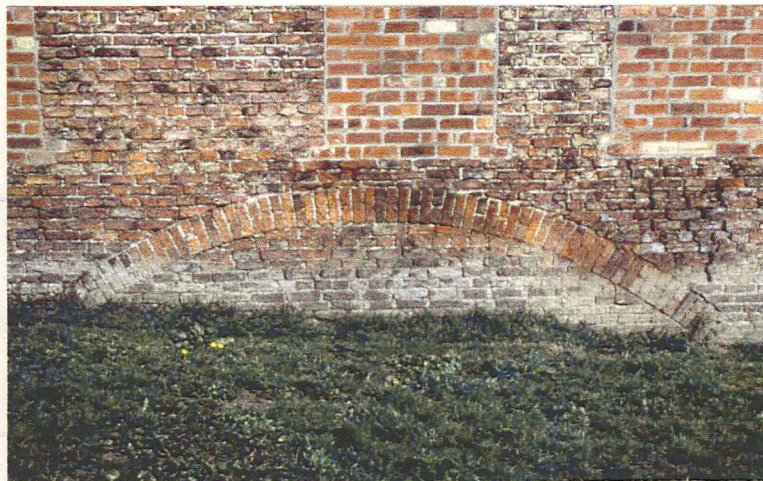
Plate 10 - Detail of the infilled eastern arch for access to water wheels, looking north
