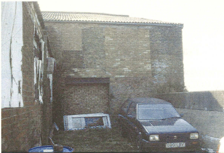
Plate 14 - Partial view of the north elevation showing blocked doorway with steel lintel over, looking south
