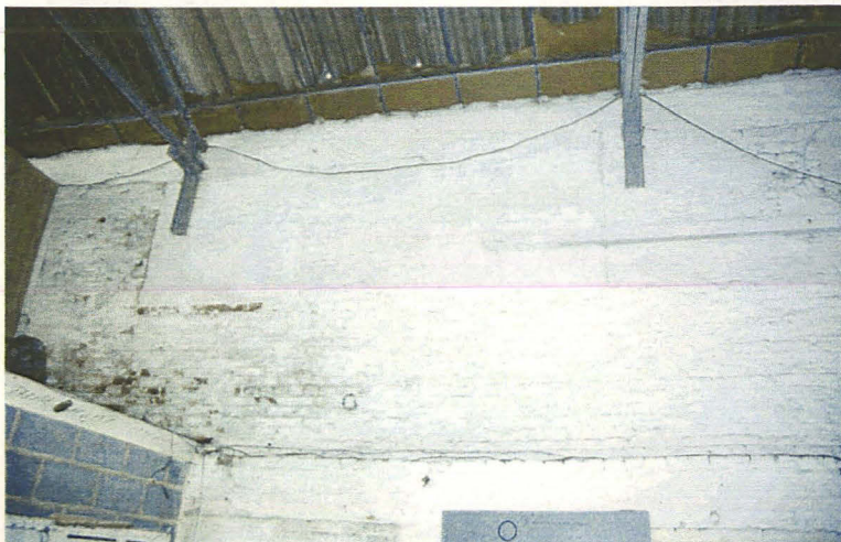
Plate 7 - Interior view of the north- ern wall showing blocked windows and part of a two storey office (left), looking north
