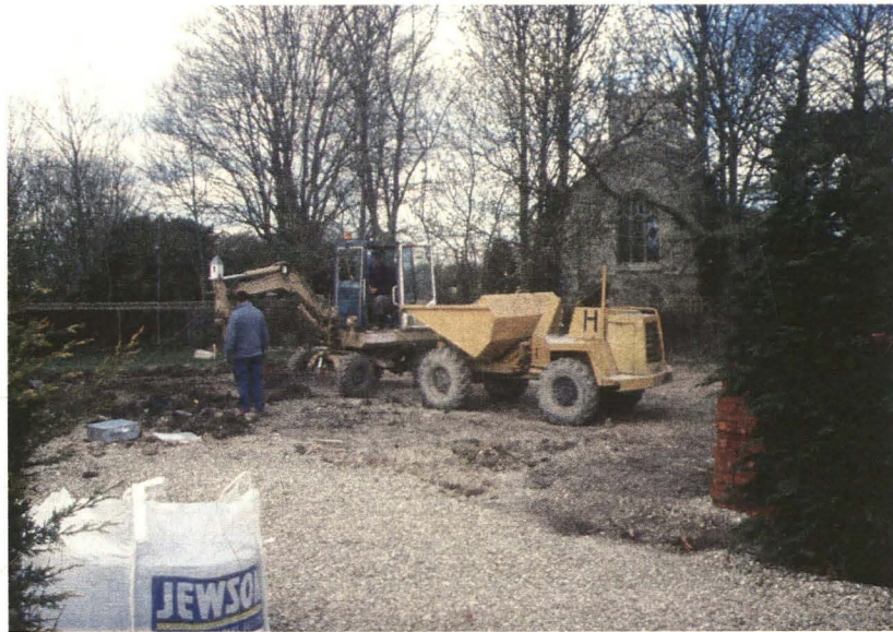
Plate 1 - General view of the development area, looking west with St. Mary's church in the background
