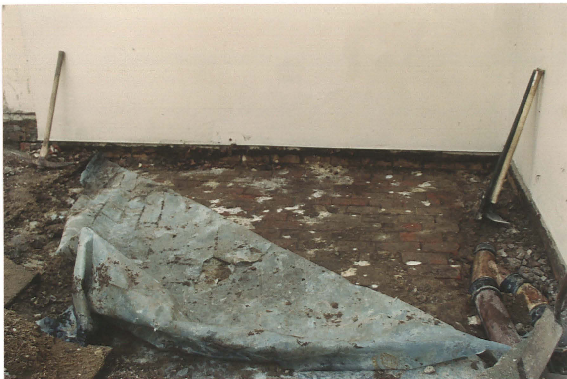
Pl. 5 Buried brickwork of the cellar roof, beside the modern entrance to the house (looking east).
