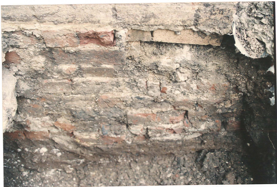
Pl. 4 Brickwork foundations of north wall of cellar, overlain by later brickwork of existing wall. Trench A, looking south.
