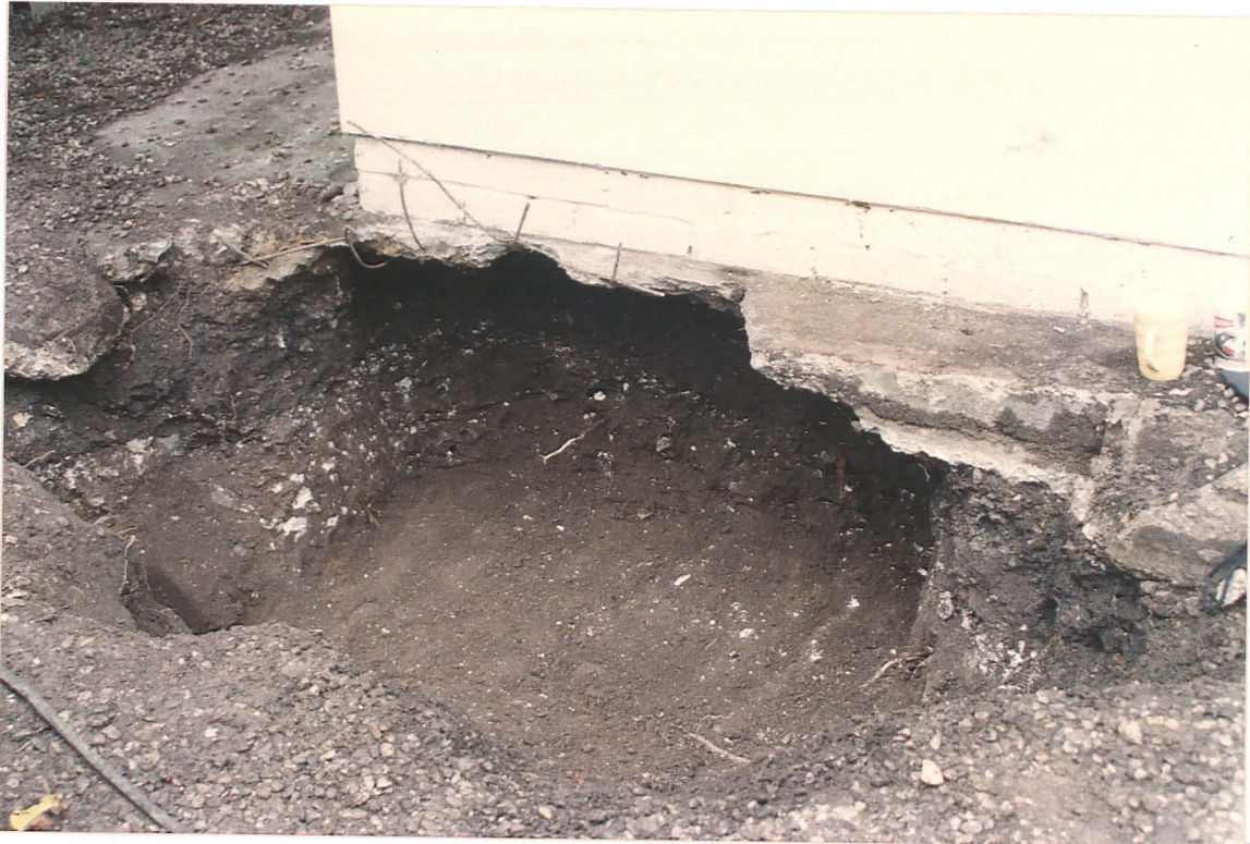
Pl. 9 Trench G at the NW corner of the garage, showing topsoil and subsoil layers sloping down to the south as fill of a linear depression. Looking NE.
