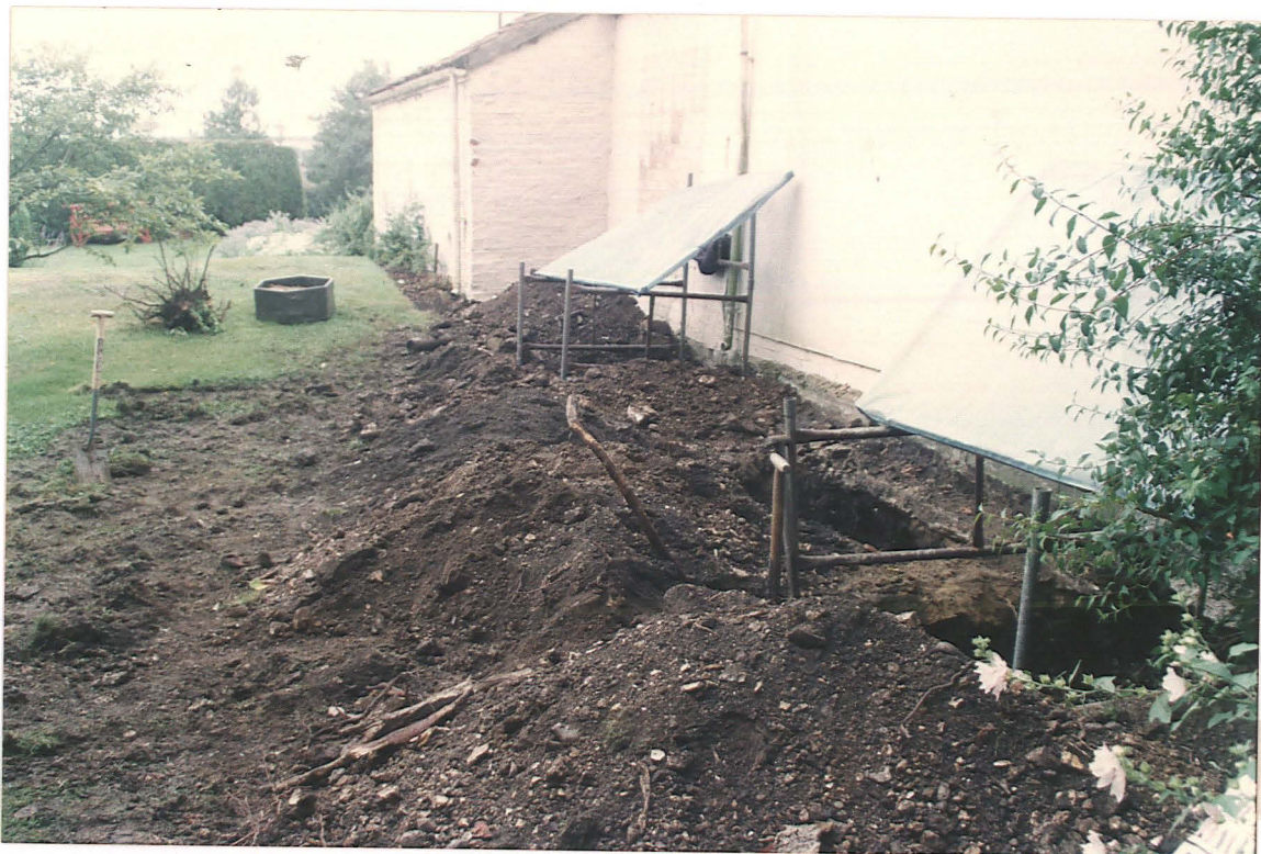
Pl. 10 Underpinning trenches H, J and K (under shelter) to the east of the garage (looking south).
