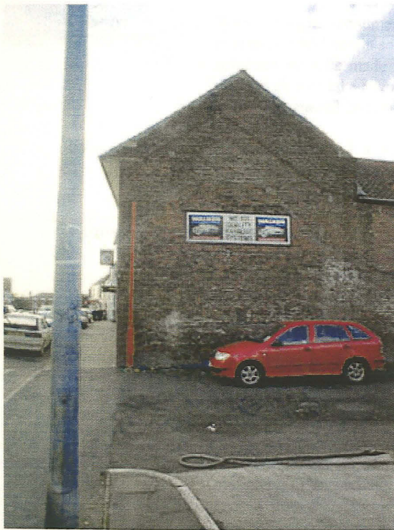
Plate 2 - View showing the roof scars from a previous building at the site, looking west
