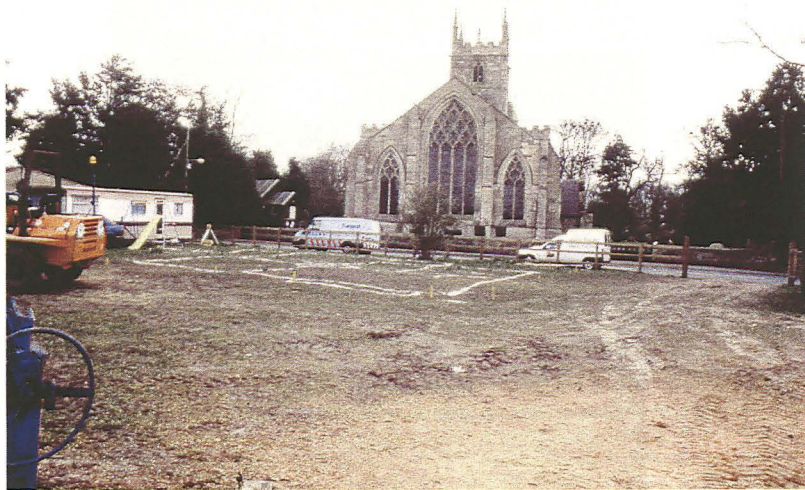
Plate 1 - General view of the development area, looking east towards St. Michael's church
