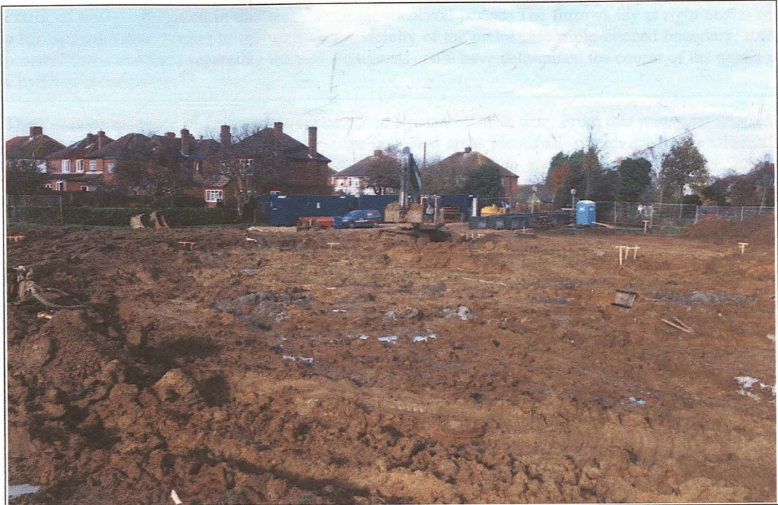
Plate I – General view of work in progress on the Day Care Centre (looking north-west).
