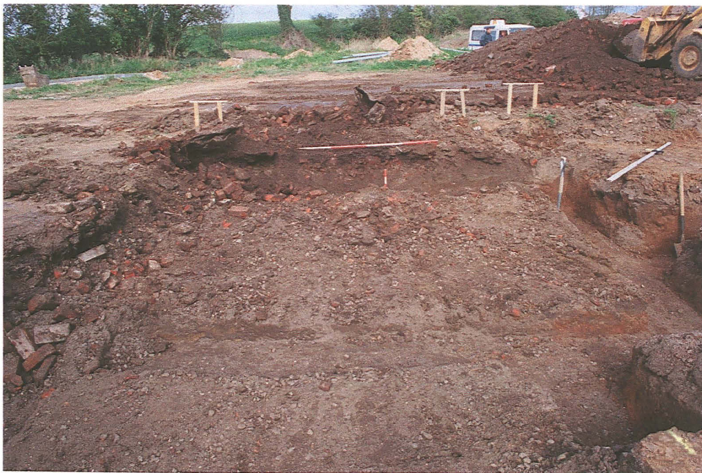
Pl. 2 Excavation of the northern third of the site illustrating the extent of the rubble infill (facing north-east). Scales 2m and 0.5m.
