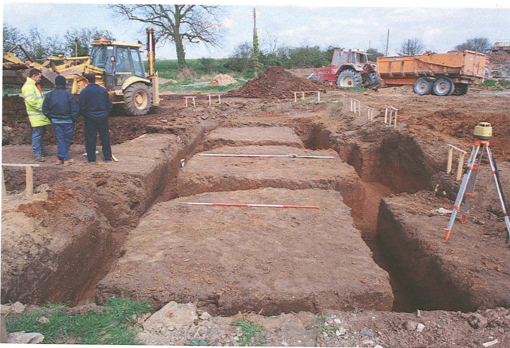
Pl. 4 View of the eastern half of the excavated foundation footprint of Plot 4 (facing north-east). Scale 2m.
