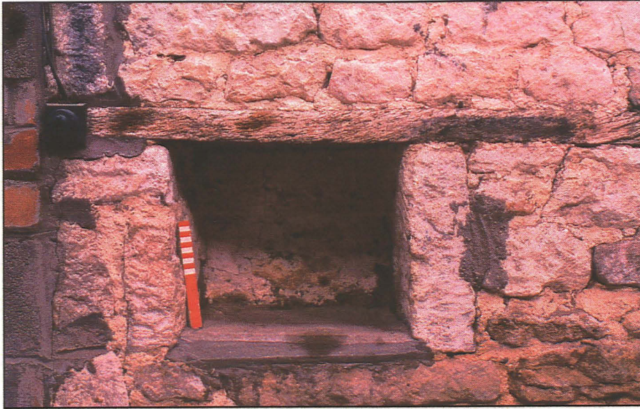
Pl. 4 Stone and timber built cupboard from north wall of barn. (Scale 20cm) Looking north.
