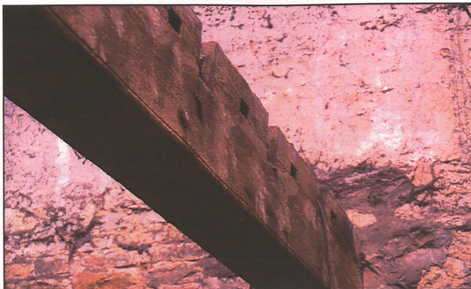
Pl. 7 Re-used beam from ceiling of Room 1. Note smaller un-used mortices, and beading on lower corners. Looking north east
