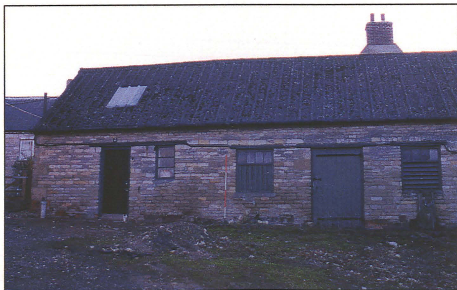
Pl. 9 Northern end of western elevation. None of these interiors could be examined. Looking east.
