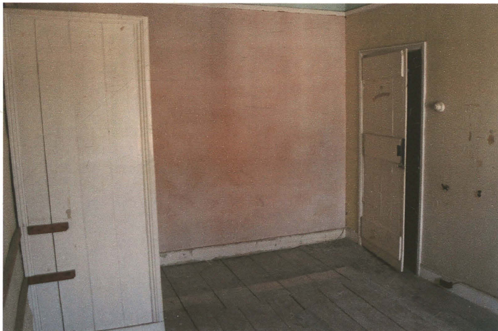
Pl. 19 Second floor south bedroom. Note replaced floorboards along west wall. Looking west.
