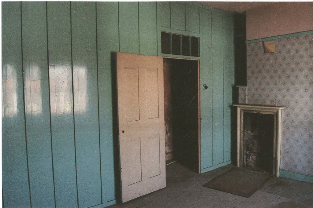
Pl. 16 Second floor middle bedroom. Note inserted panelling to form corridor access to south bedroom and fireplace on north wall (surround removed).
