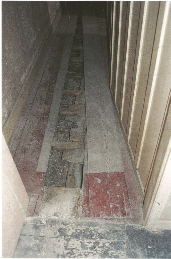
Pl. 18 Second floor corridor with floorboard removed revealing earlier floorboards, partially sawn off. Looking north.
