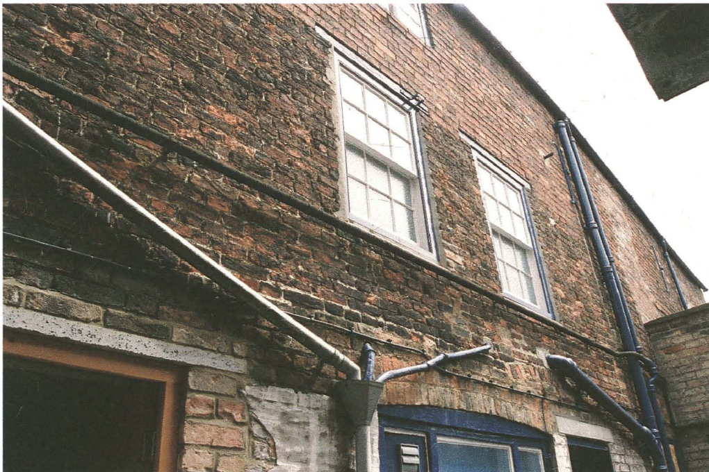
Pl. 5 Rear elevation looking southeast, showing red brickwork of upper storey and new first floor sash windows.
