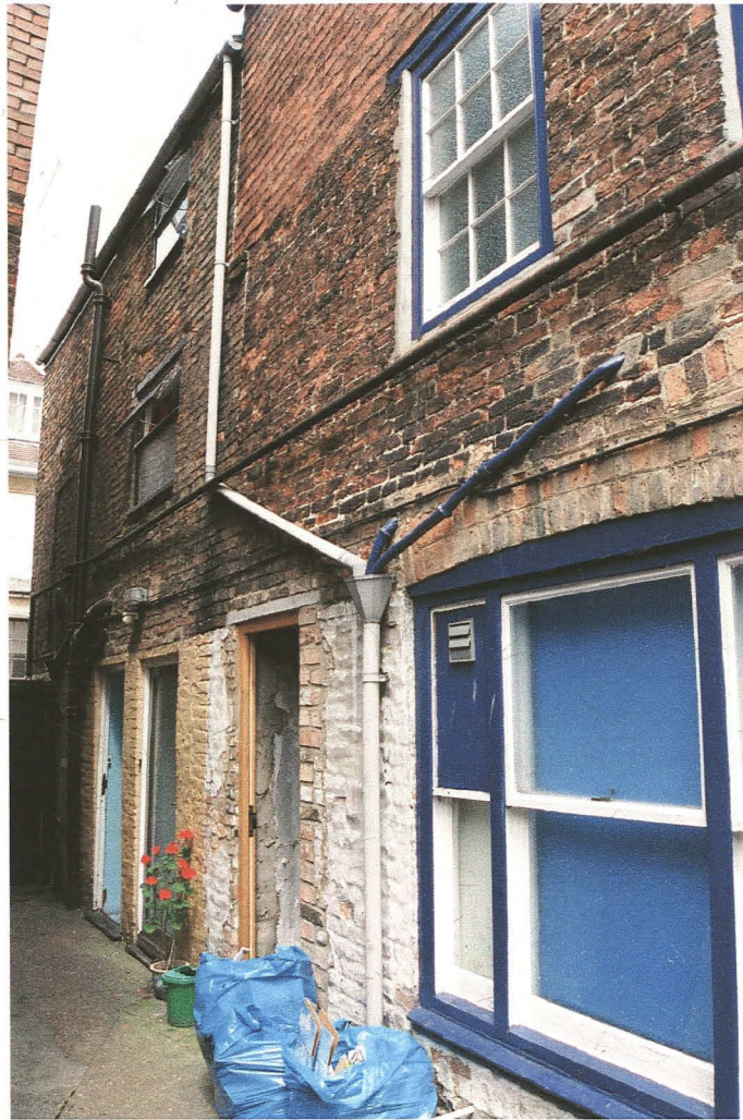
Pl. 4 Rear elevation north end, showing inserted door and vertical joint in brickwork (right of white drainpipe). Note red brickwork of upper storey.
