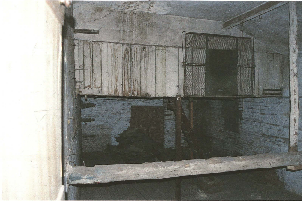
Pl. 14 Rear room straddling the first and second storeys, with mezzanine accessed by a ladder. Looking south. Note modern blocking in south wall which would have led into the adjacent property, Lloyds Chemists.
