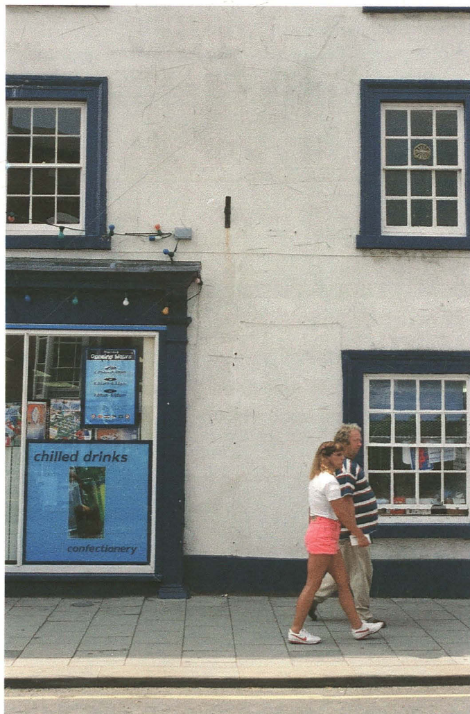
Pl. 2 Front elevation detail showing crack in render to north side of shop front, rising above first floor window.
