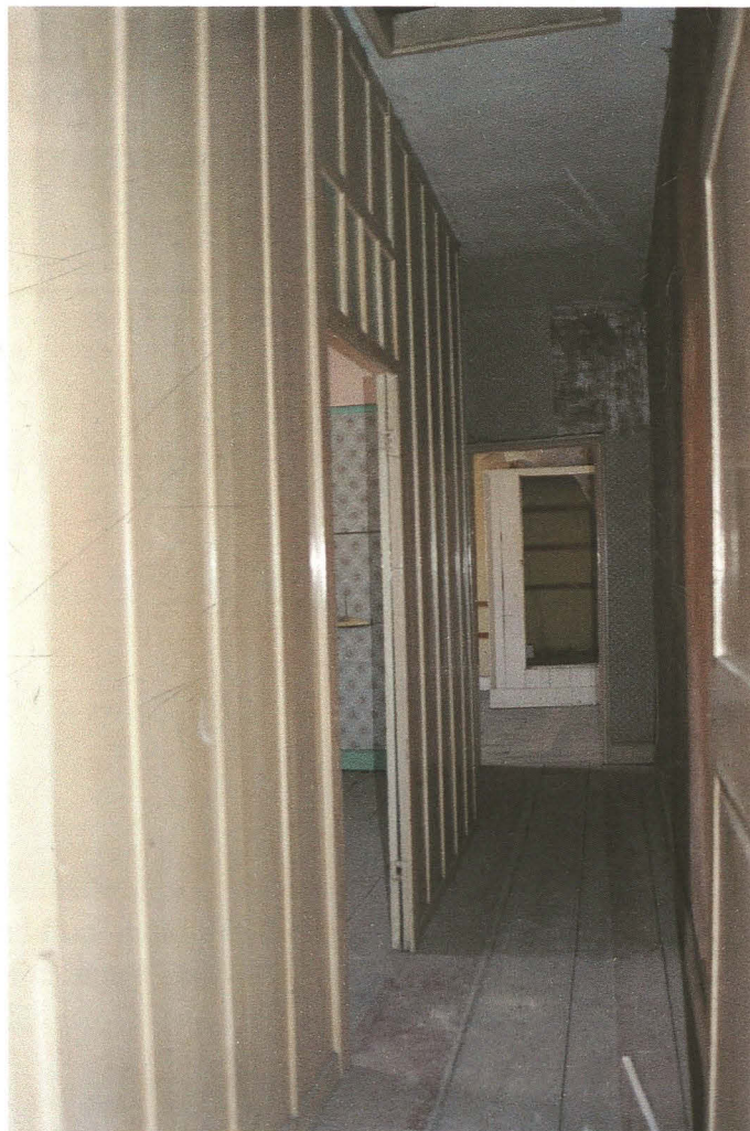
Pl. 15 Corridor leading to south bedroom. Note wood panelling of central bedroom west wall to left.
