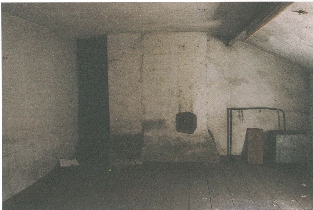
Pl. 13 Second floor rear bedroom, looking south, showing firestack with inserted soot box and opening to left of firestack which overlooks the inaccessible rear large room.
