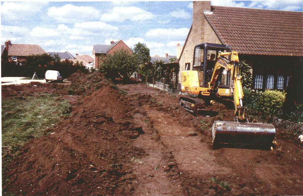
Plate 1 General view of the site showing topsoil stripping in progress, looking north
