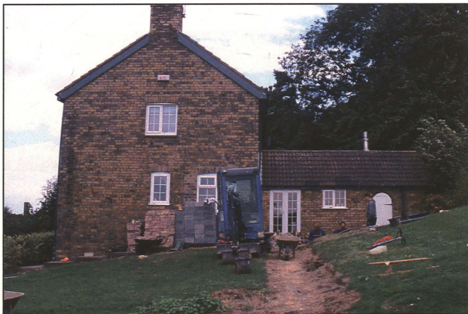
Plate 3: the west side of the existing house (area of excavation to the right), showing the slope of the surrounding ground.
