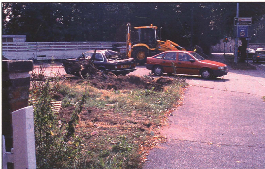
Plate 2 (right): General shot of the development area taken during the machining of the evaluation trench, looking south-east.
