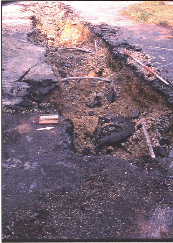
Plate 4 (left): General view of the trench excavated in the preferred area, looking south-west. The fuel tanks (covered with concrete) and associated pipework can be seen throughout.
