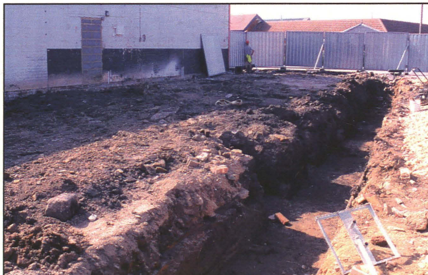
Plate 6 (left): General view of the site on completion of the machining, looking north-west.
