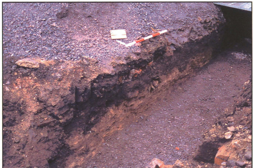
Plate 5 (right): North facing section of the foundation trench for the north wall of the new building, looking south-west.
