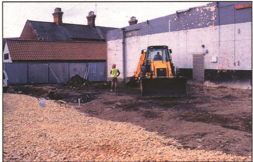
Plate 2 (right): General shot taken during the machining of the foundation trenches, looking south-west.
