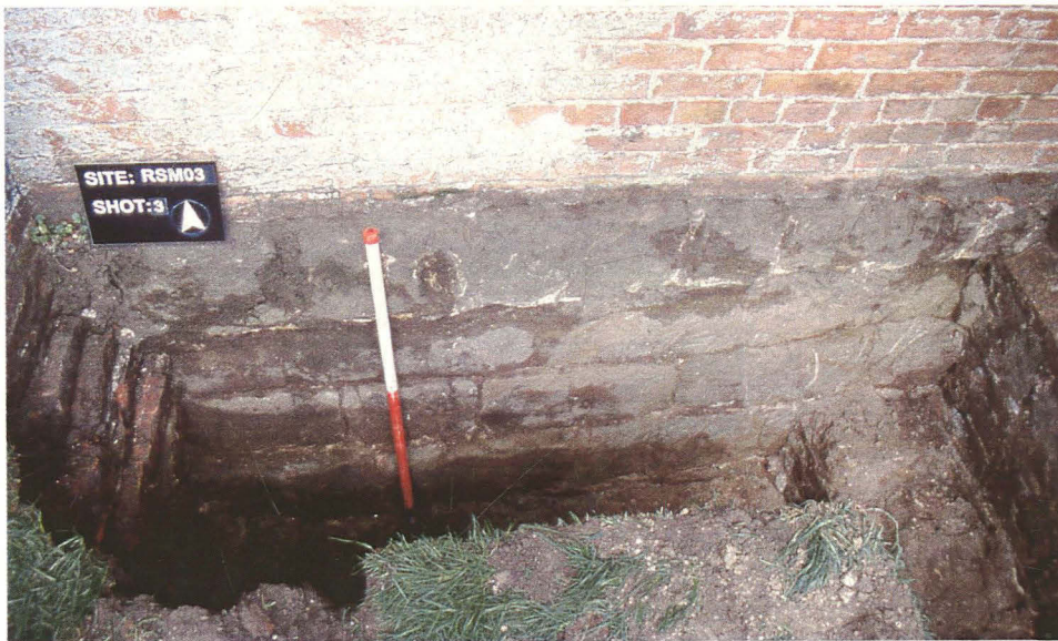
Plate 2 Section 1 looking north, showing foundations of the south wall of the tower.
