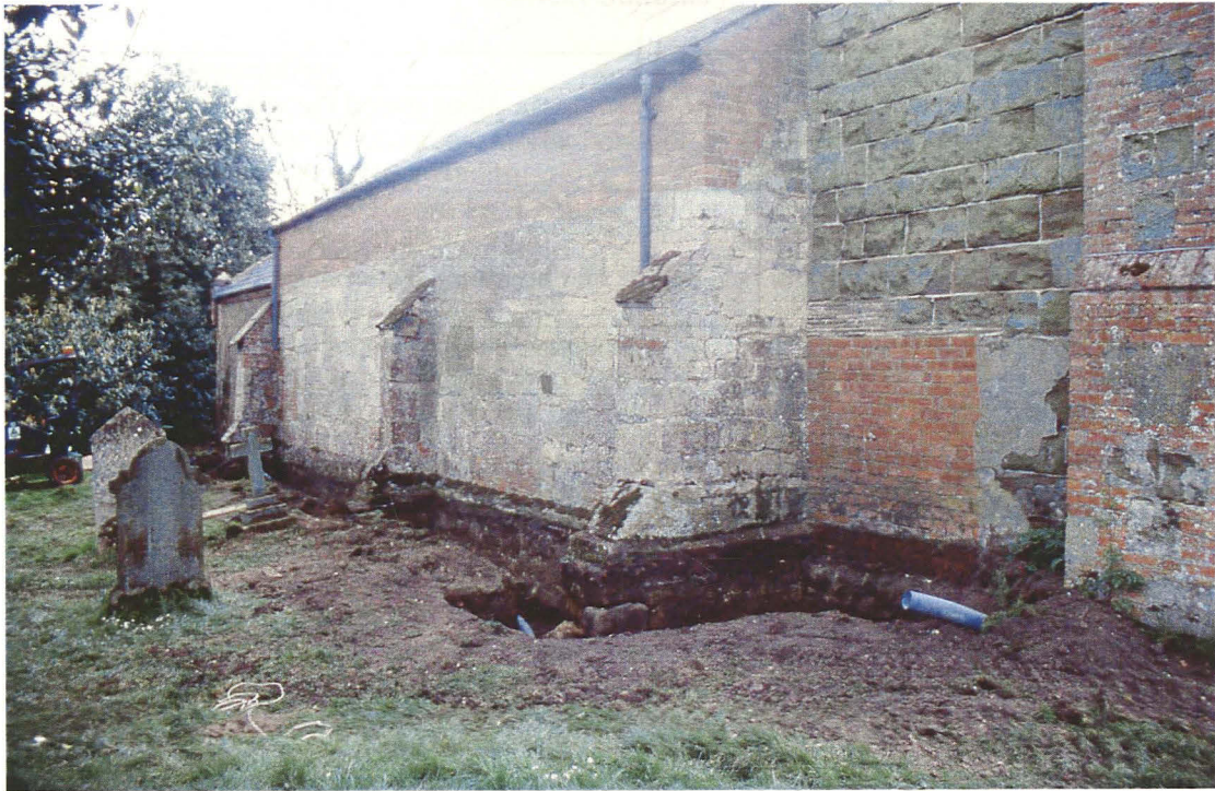
Plate 6 General view of the trench along the north wall of the nave, looking southeast.
