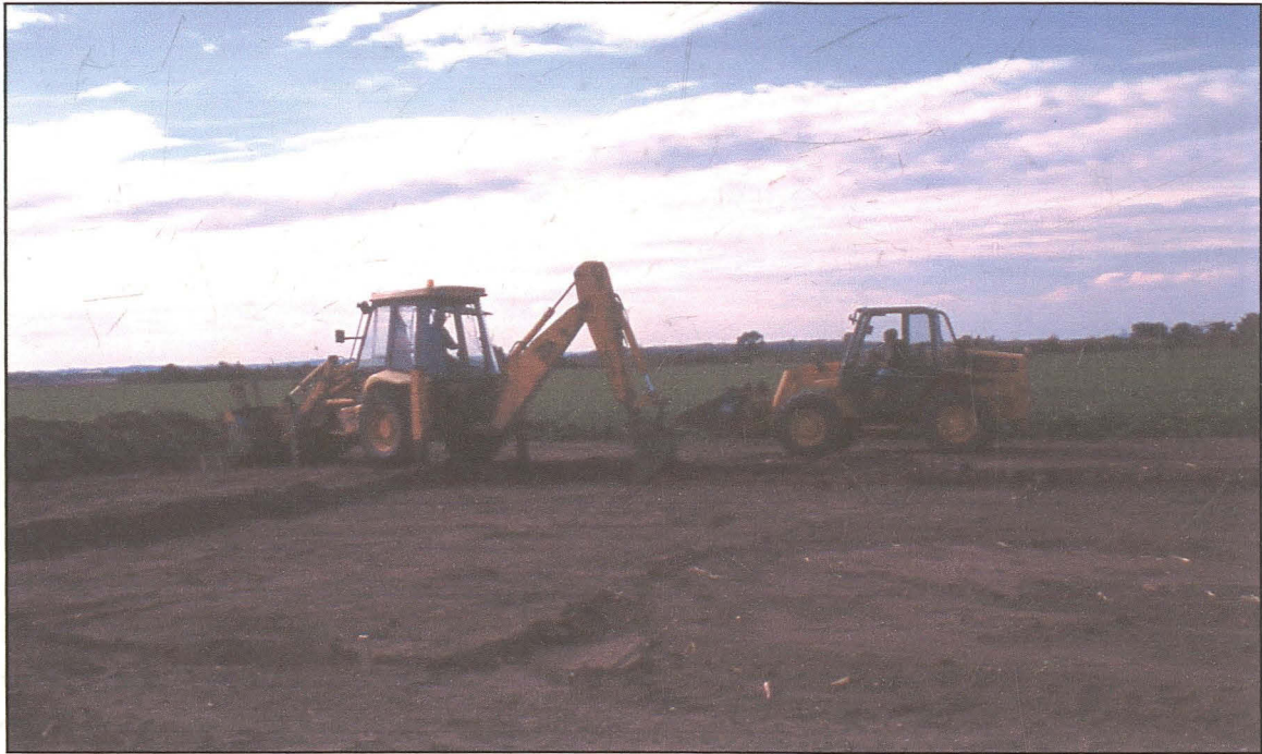
Plate 1: General shot of site, looking WSW: excavation beginning for the foundation trenches of the house plot (Trench 1).
